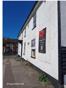
Unauthorised signage removed, temporary signage attached to the exterior of the building, also unauthorised.
