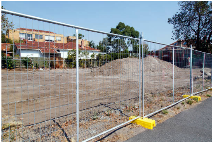
Heras Fencing Image.
