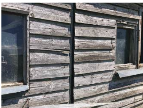
Photograph 11: Example of lifted wood cladding
