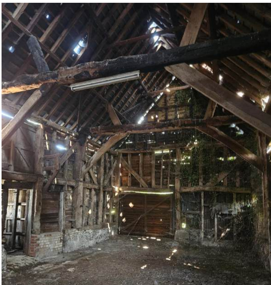
Plate 27: General view looking towards eastern end of Barn 1 showing blackened roof trusses
