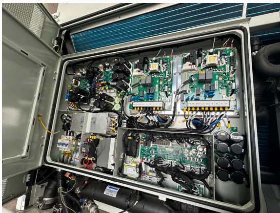
Figure 6-8 Chiller auxiliary panel
