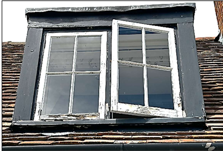
Figure 15. Rot to the base of window 12 (rear wing, south roof slope)
