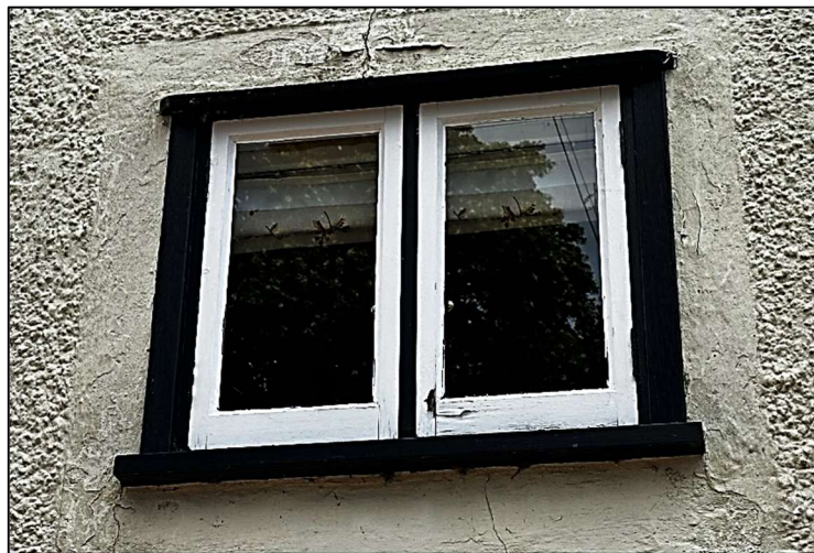
Figure 16. Window 20 (north gable end of main range, 1 st floor). Rot to base of window next to joint.
