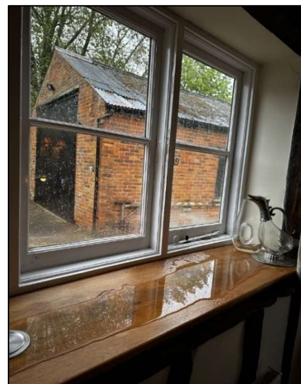
Figure 18. Window 4. Water ingress sitting on window ledge
