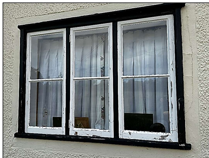
Figure 14. Window 2 (front elevation, ground floor centre). Peeling paint and rot to bottom part of window
