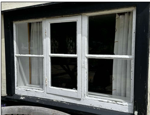
Figure 17. Window 5, south gable end of front range. Rot to base of window.
