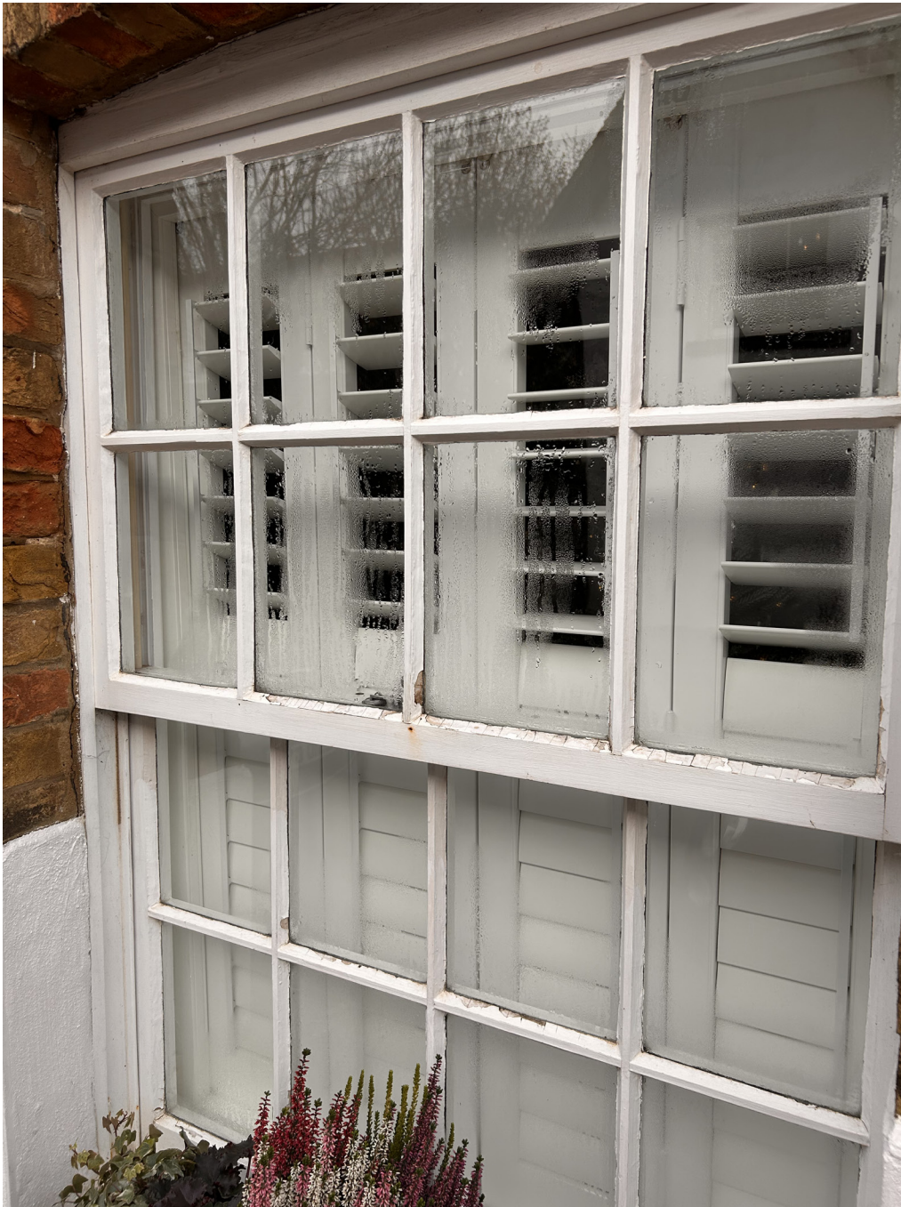
Existing sash windows, damaged, to be replaced
