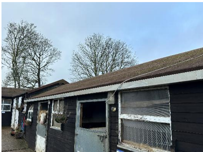
Plate 7. Felt stable block roof.
