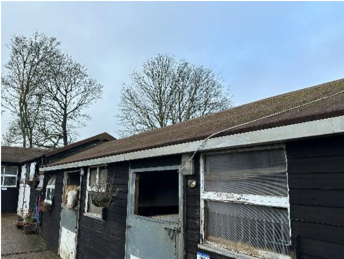
Plate 7. Felt stable block roof.
