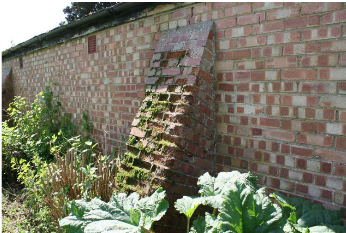
Detail of the NE elevation of the Workshop. Note the cracking and spalling.
