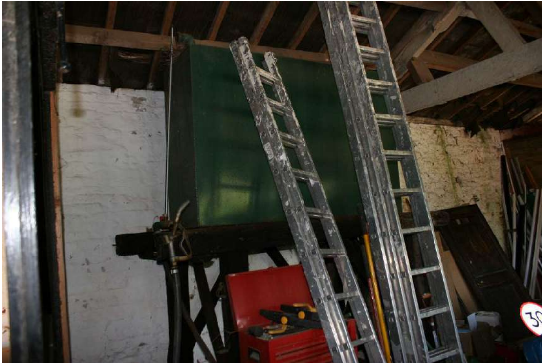
Diesel oil tank in the NE bays.
