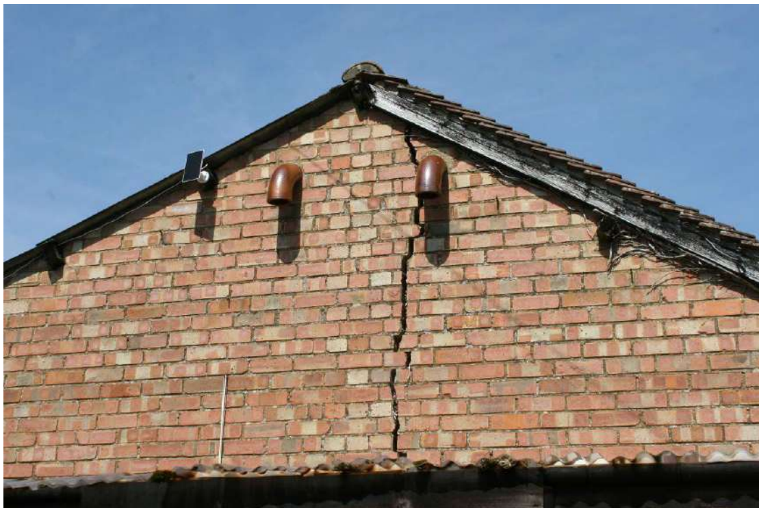
The SE elevation has a serious crack. The vents are sewer pipes.
