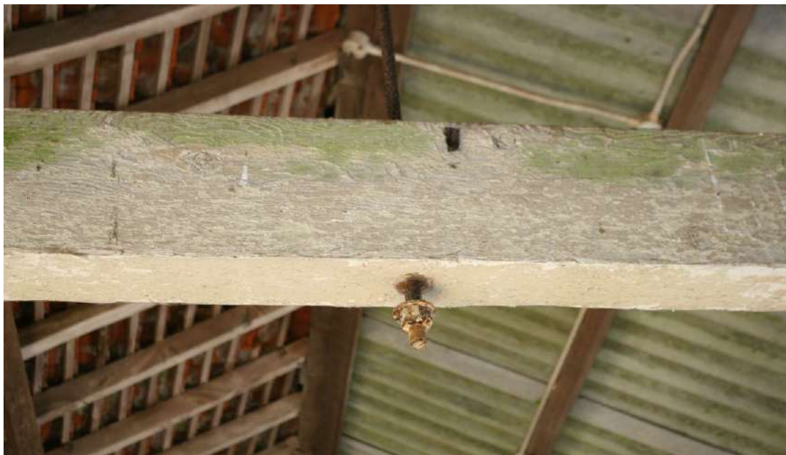
Detail of the king bolt showing the sag of the roof.
