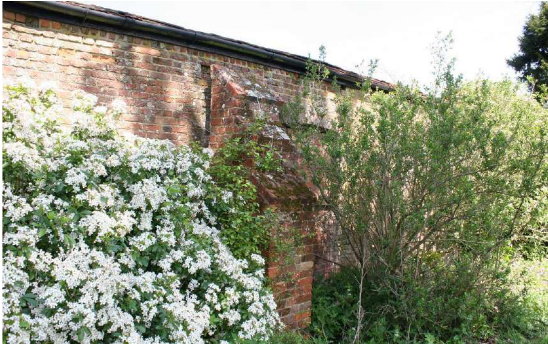
The wall has shifted away from the buttress.
