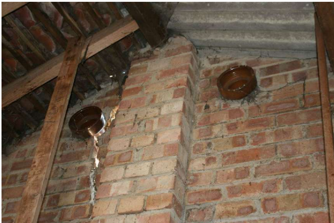
Air ducts made from sewer pipes. One has started off a massive crack.
