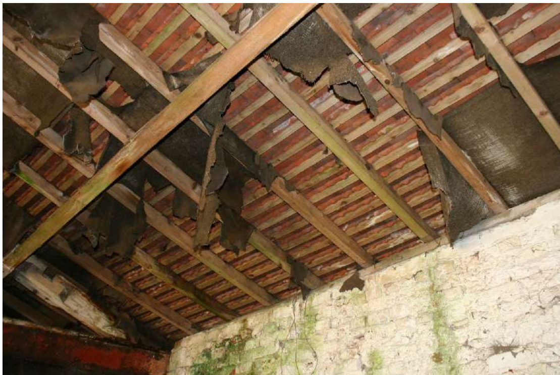
Detail of the failed asphalt membrane.
