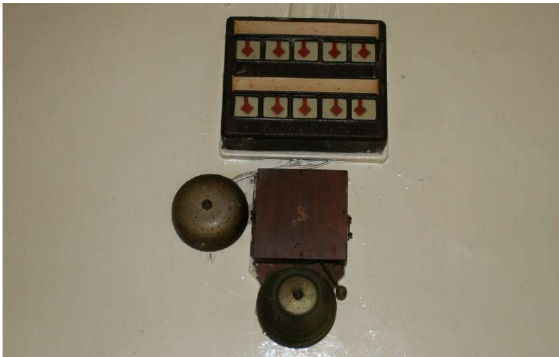
MC20th electric service board and doorbells.
