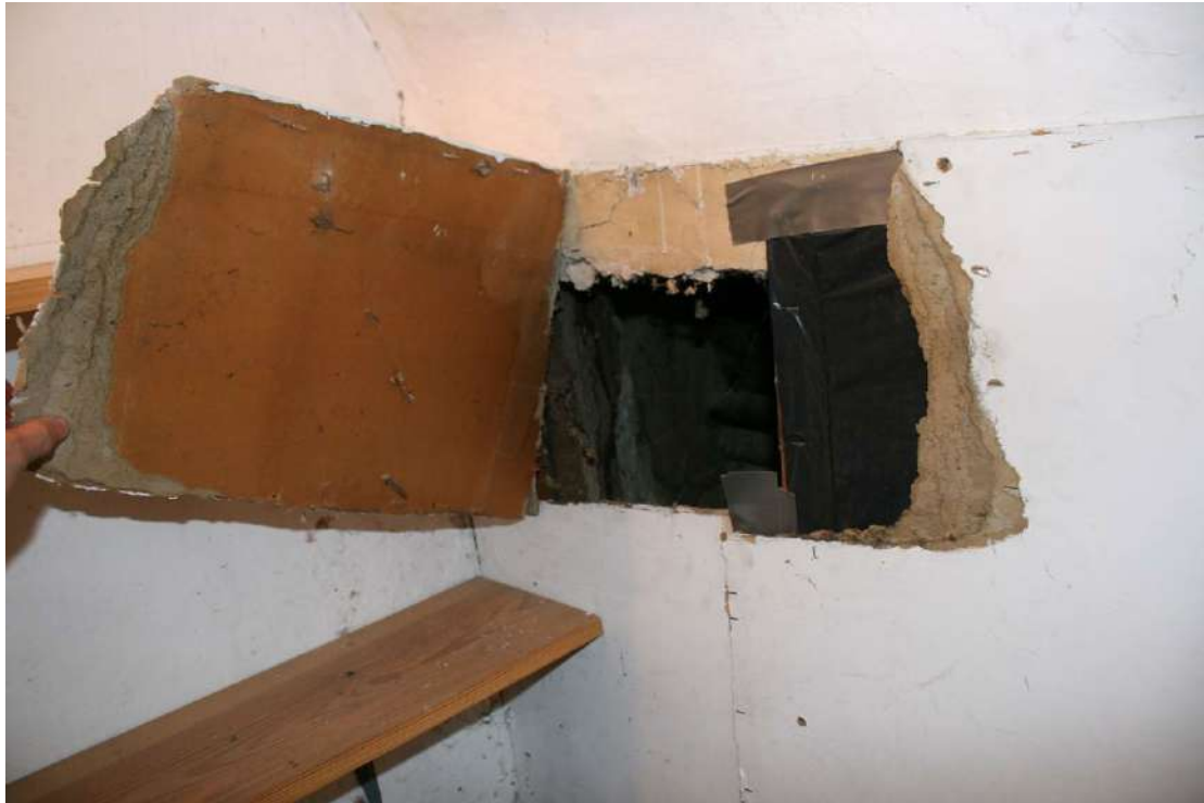
A section of hardboard panelling has been pulled back to get at the pipes.
