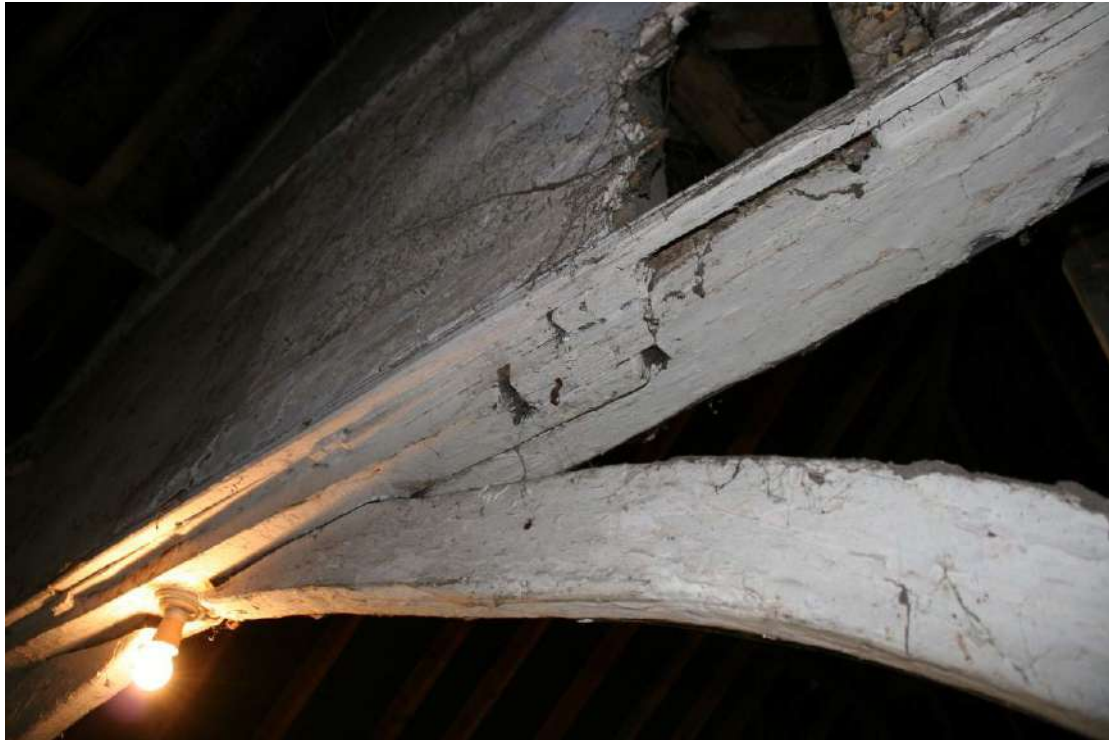
The east side of the partition wall showing the failing scarf joint.
