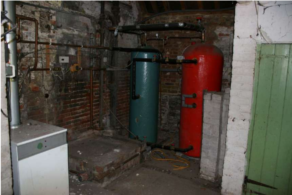
There is a modern boiler system that replaces the 1939 boiler.
