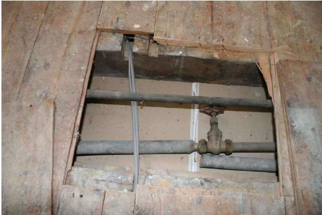
Lifted boards in the WC show the lead pipes and the plasterboard ceiling below.
