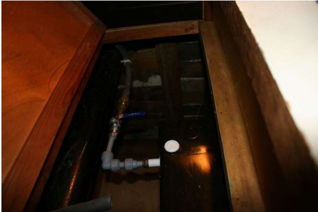
Plywood closet to conceal the cistern for Bathroom 2.
