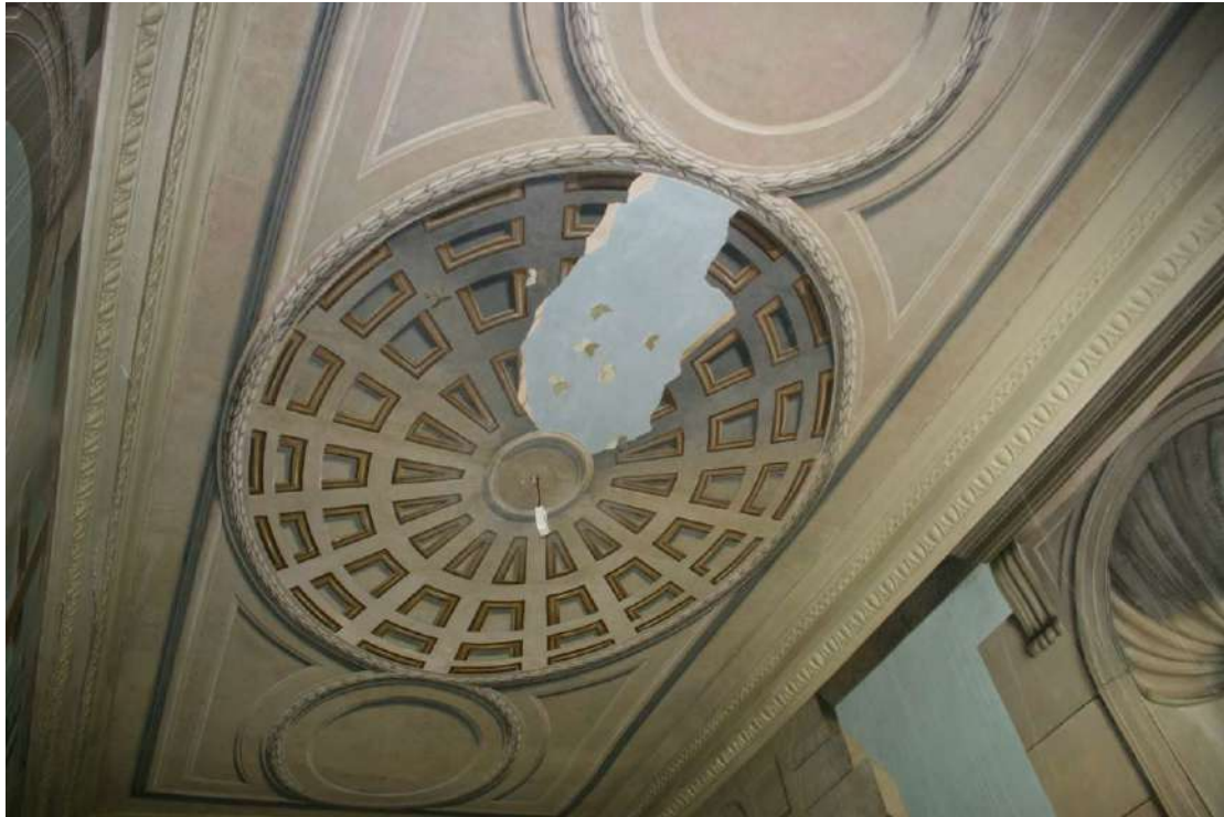
The ceiling has water damage.
