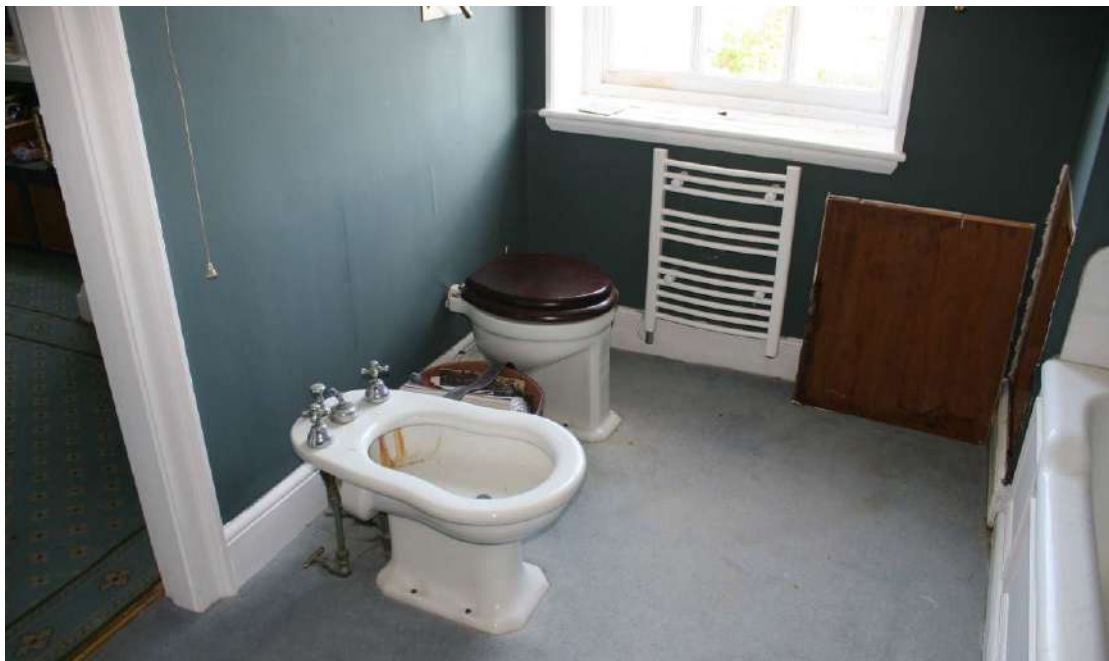
1939 original bidet and WC with original 1939 pipe work.
