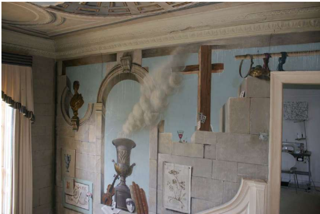
The east wall has serious cracking in the render.
