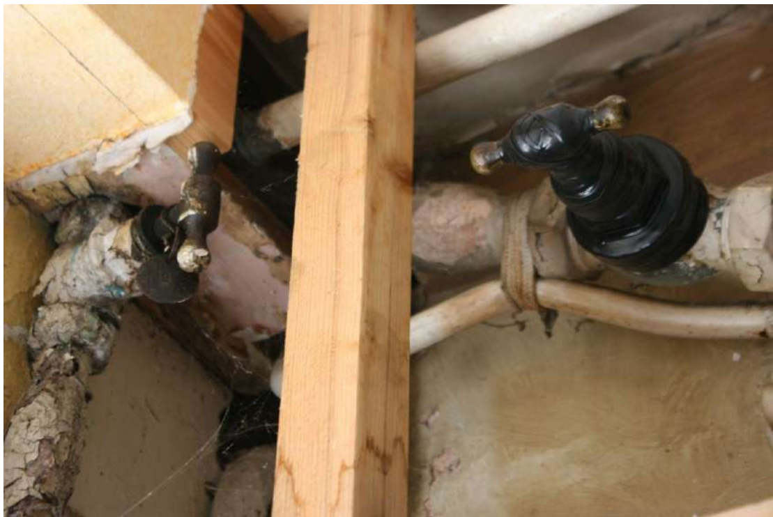
Detail of the 1939 stopcocks. One takes water from the well in the garden.
