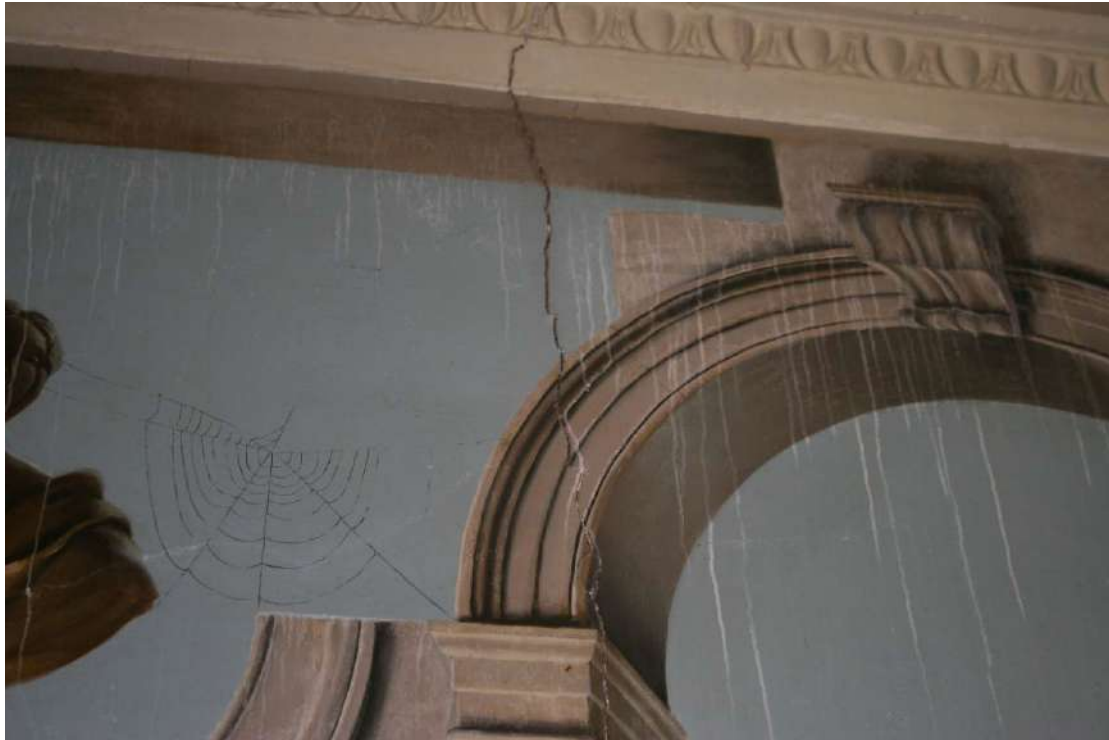
Deep visible crack in the east wall.
