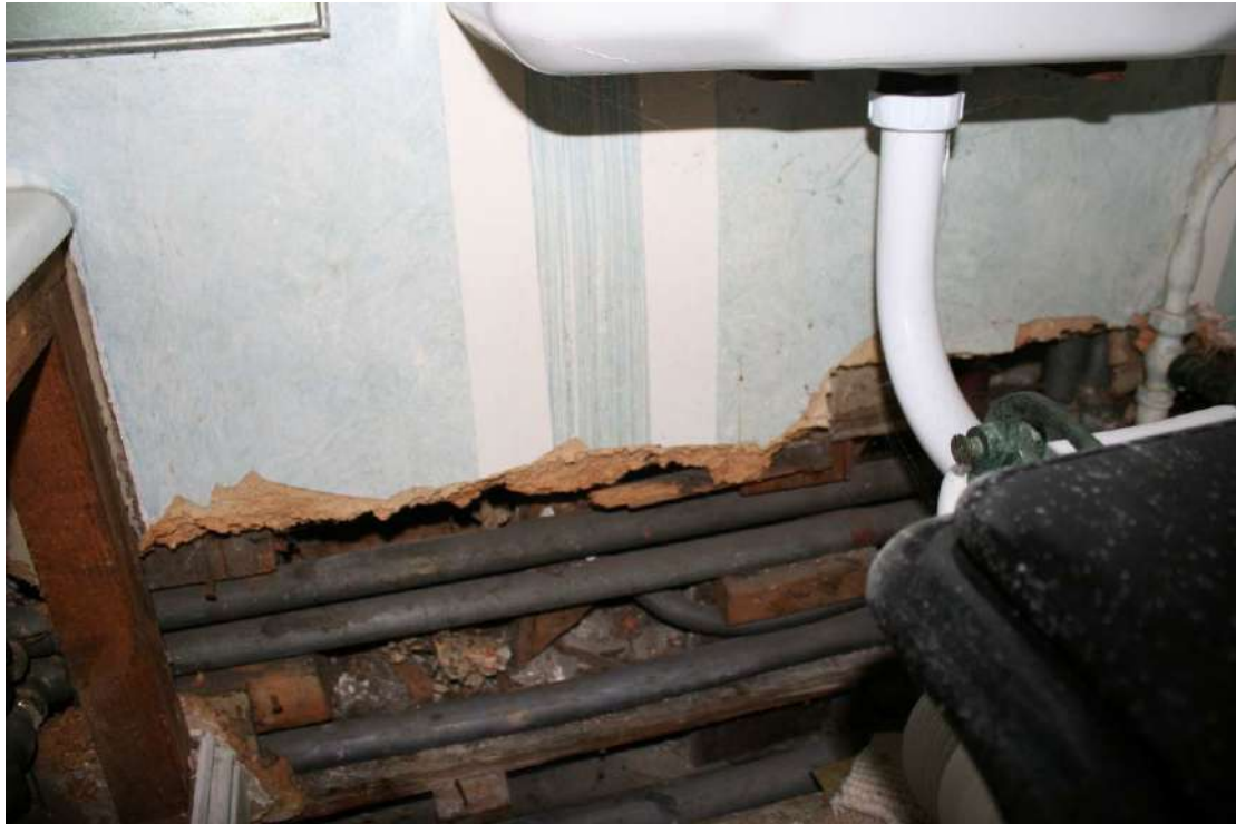
Water damaged hardboard panels concealing the lead water pipes.
