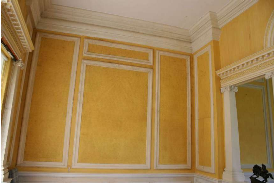
The wall panels on the NW corner wall looking N are loose.
