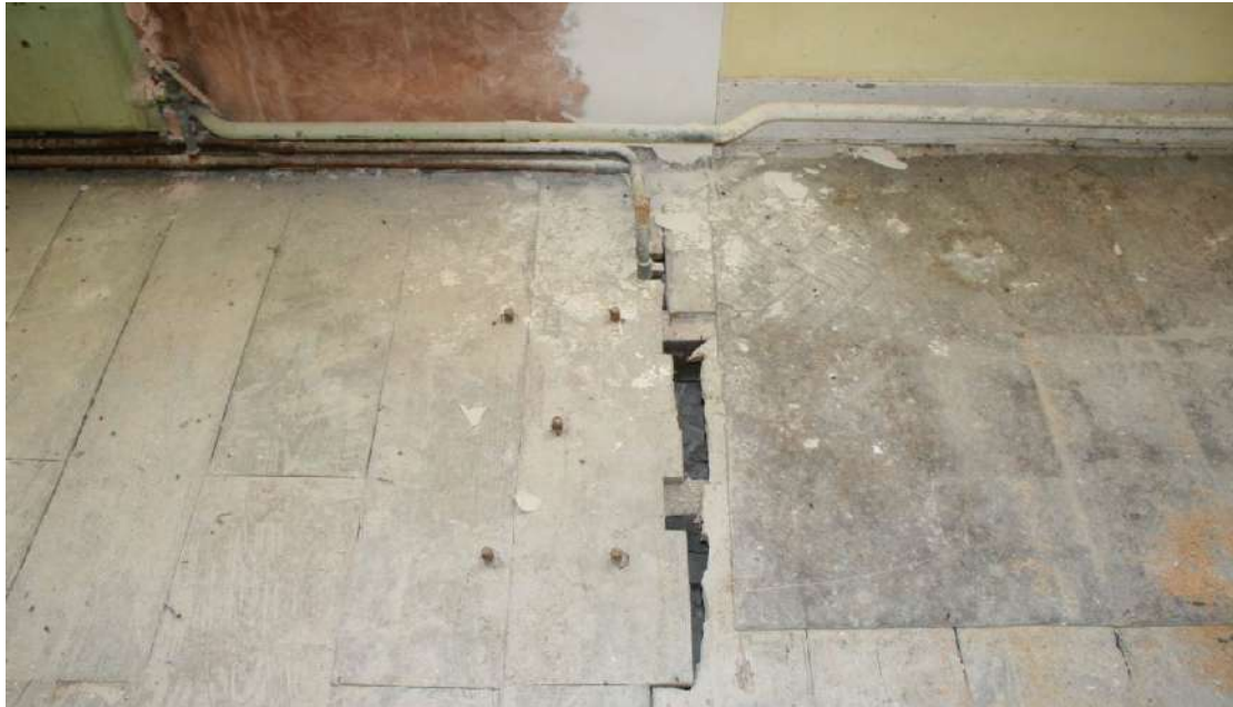
The floor has been water damaged where bath was fixed to the floor. Looking N.
