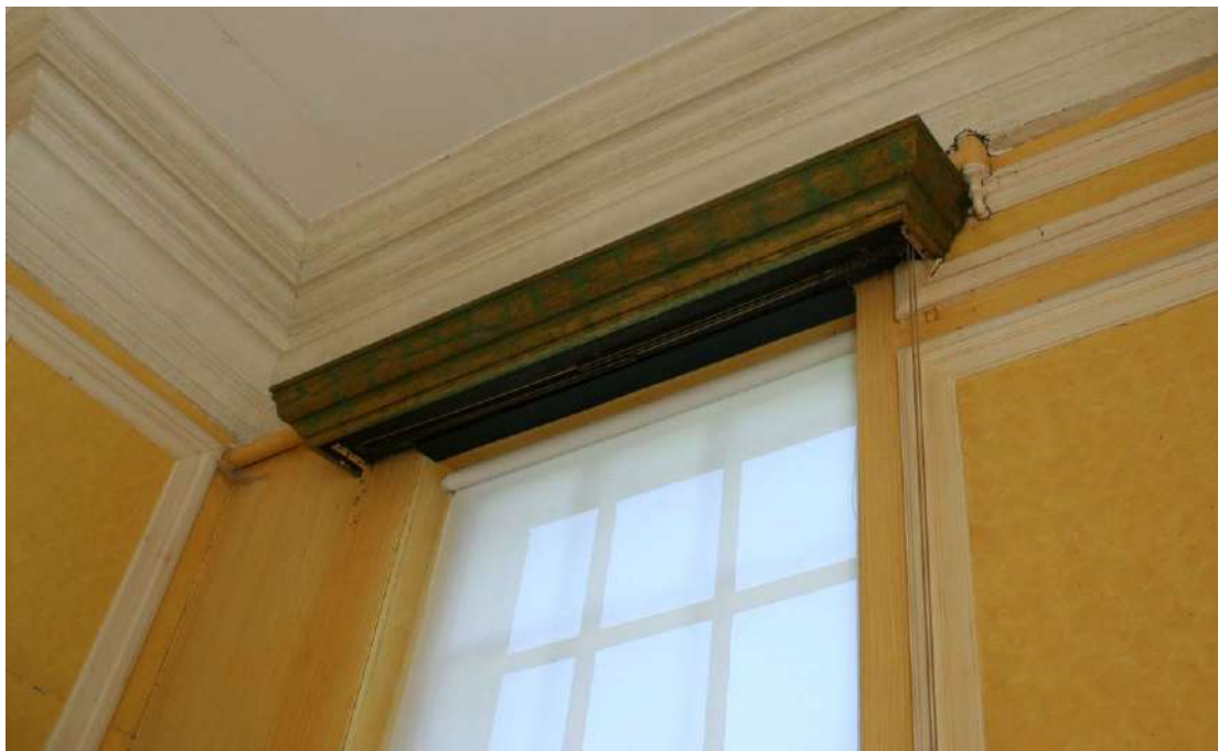
Water pipes concealed in the pelmet.
