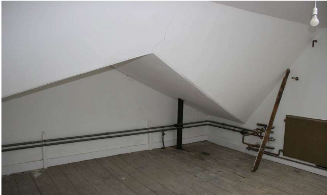
The industrial radiator in Room 7.
