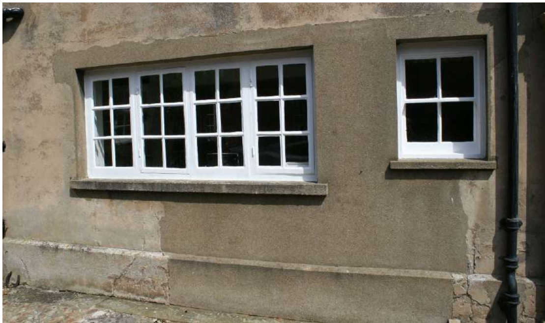
Modern repairs to the render on the ground floor.
