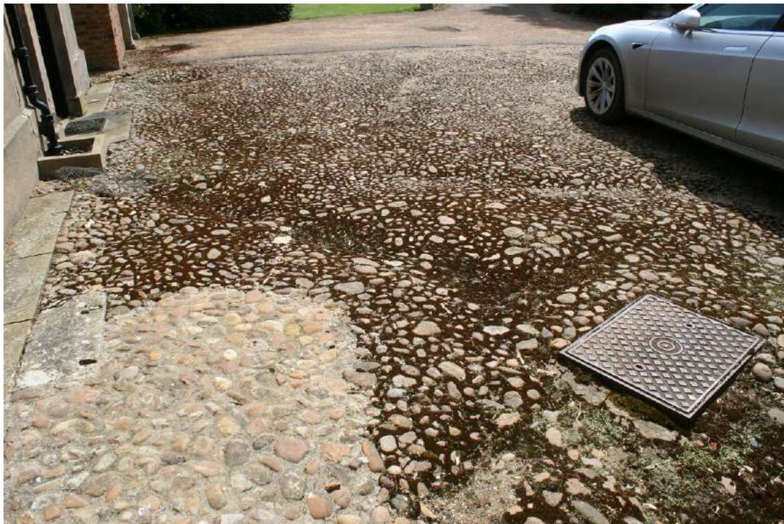
Cobbled surfaces with drainage trenches for MC20th drains.
