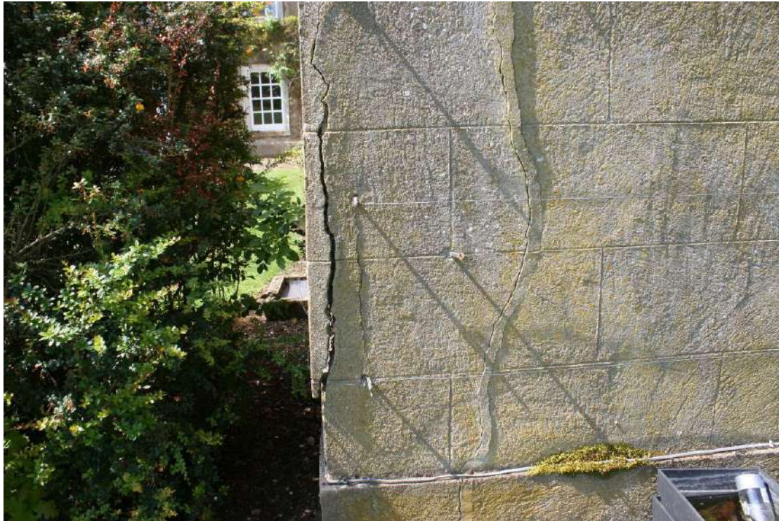
Detail of the render on the east elevation with serious cracks.
