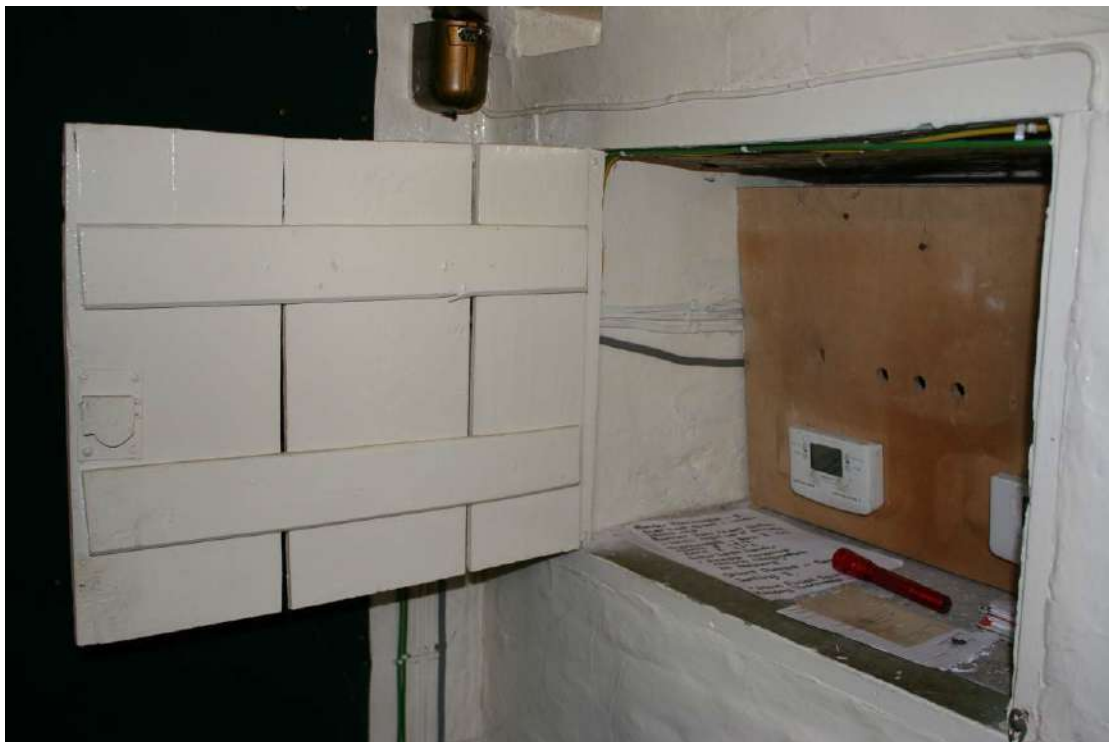
Electrical cabinet with modern heating controls.
