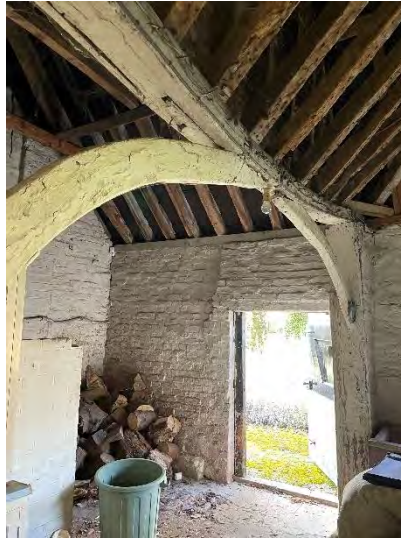
Timber brace to be repaired/strengthened
