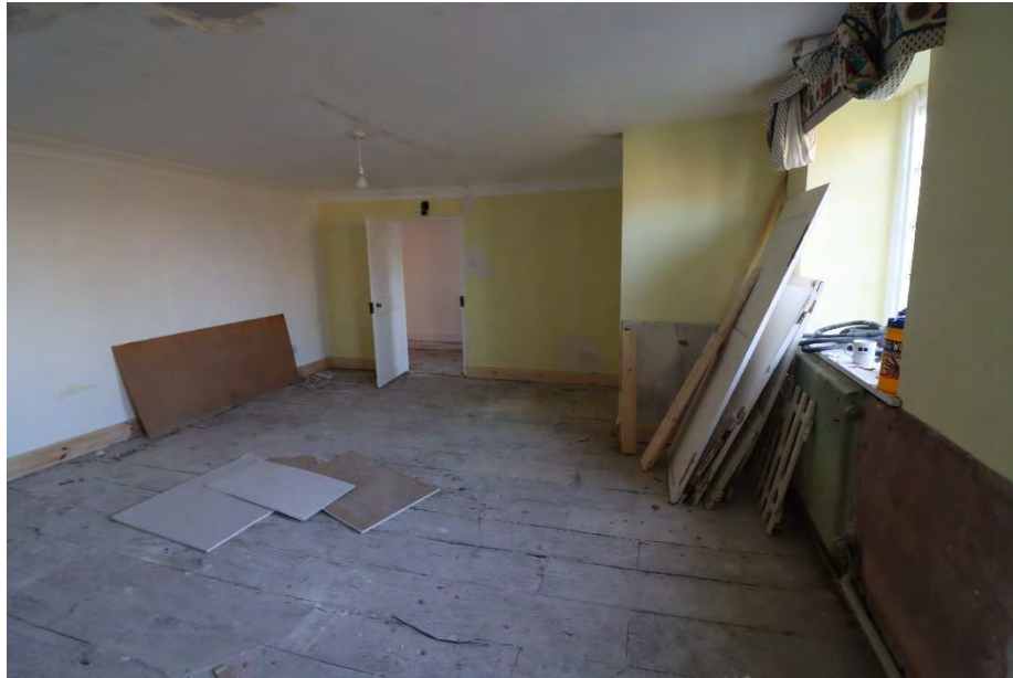
MC20th WC partitions to be removed (rhs)
