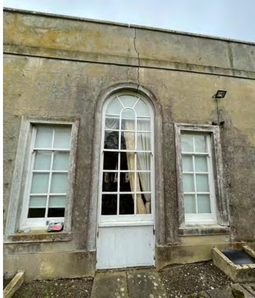
East Elevation of Music Room with vertical movement crack
