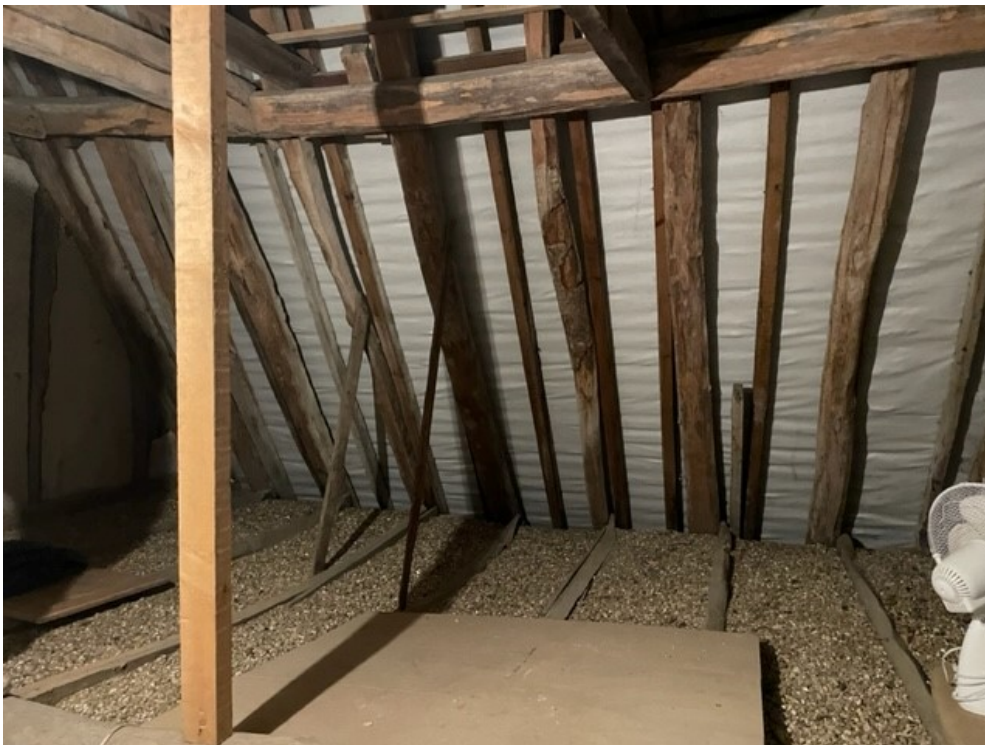
Existing loft space with supports to the bowed/sagging ceiling joists.
