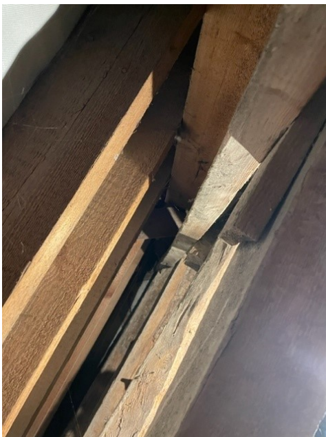
Gap between the new rafters and the old rafters
