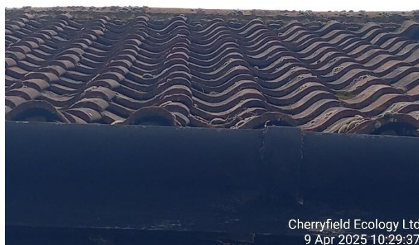
Figure 21: Lifted interlocking clay tiles.
