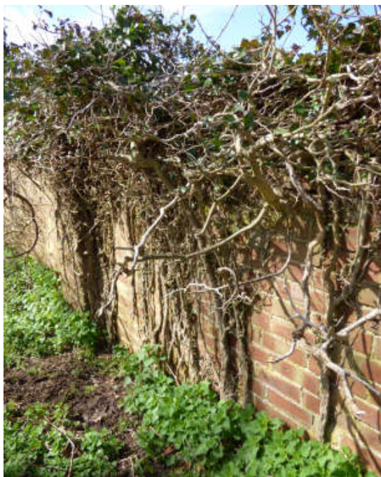
Above, extensive ivy cover to south end wall (C)
