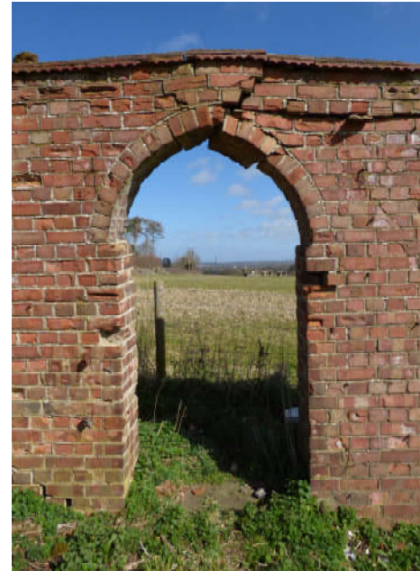
Unstable brick arch to side gate
