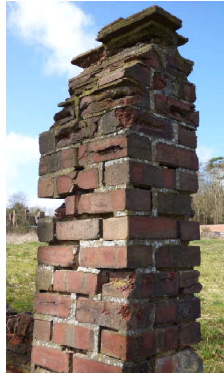
Example of extensively eroded and open jointed brickwork to piers along section (c)
