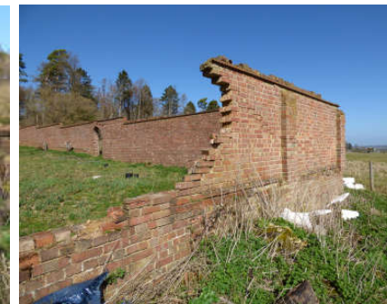
Northerly end, high wall partially collapsed
