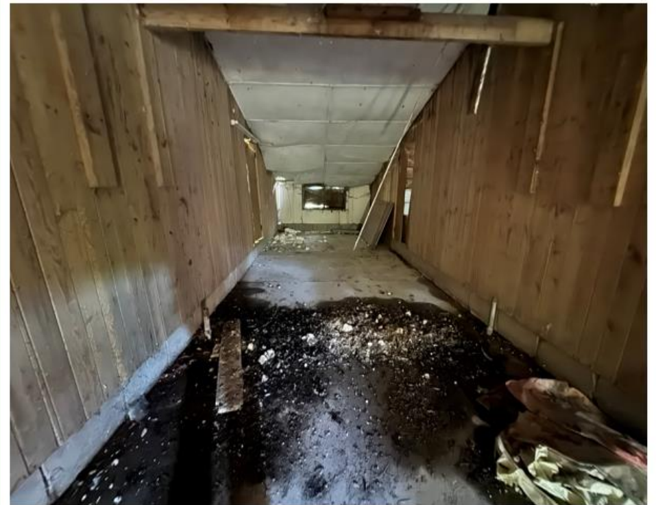
Photo No.10: Small room separating the eastern and western wings of the poultry shed (roofing above allowing water ingress)
