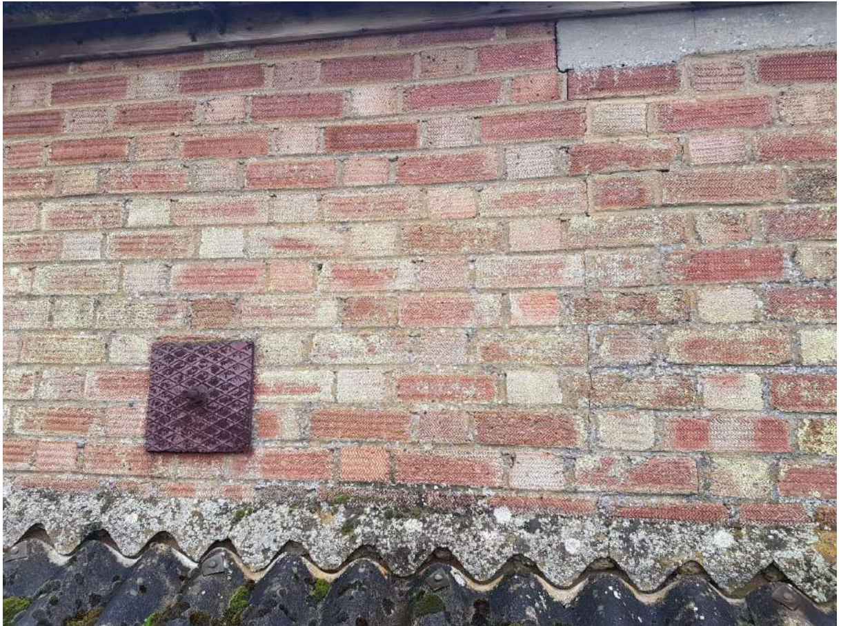
Photograph 7 – Masonry cracking adjacent Wall Plate Anchor in Barn A
