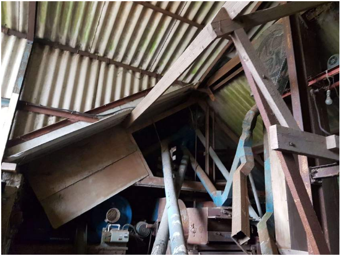
Photograph 29 – Disused Agri-plant and roof structure to Barn B
