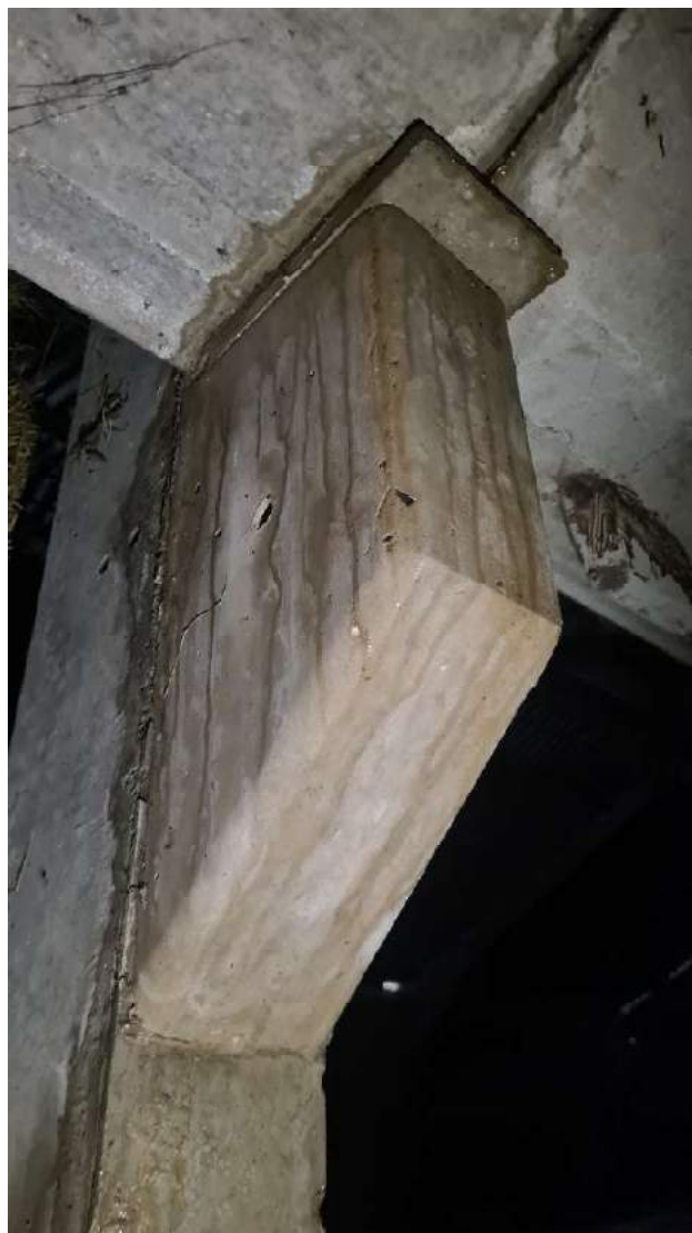
Photograph 18 – Gutter junction with water ingress
