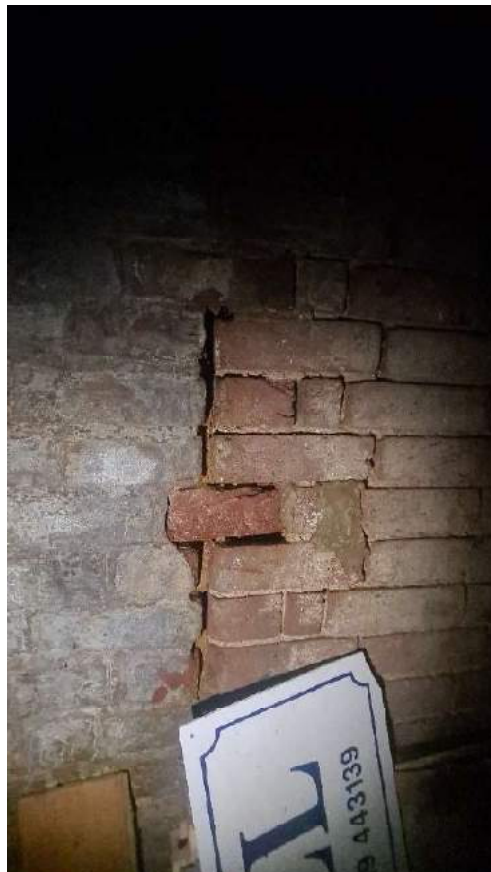
Photograph 16 – Masonry infill junction to be repaired
