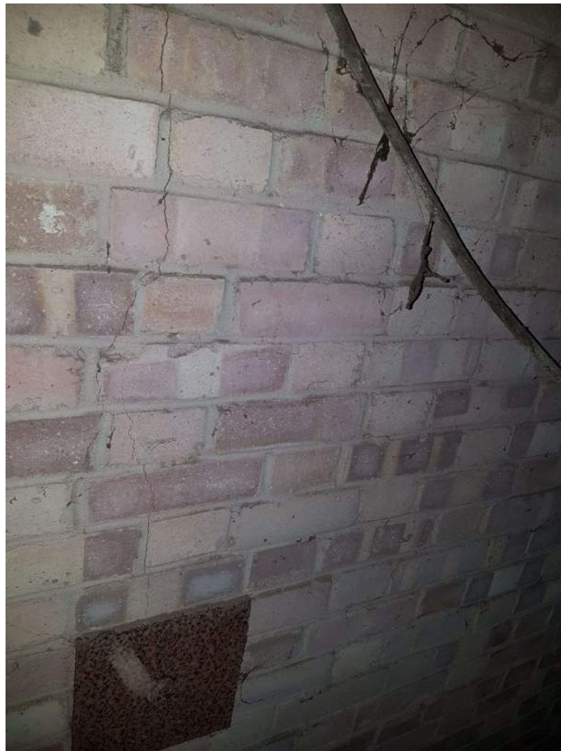
Photograph 12 – Cracking above wall anchor plate in Barn A
