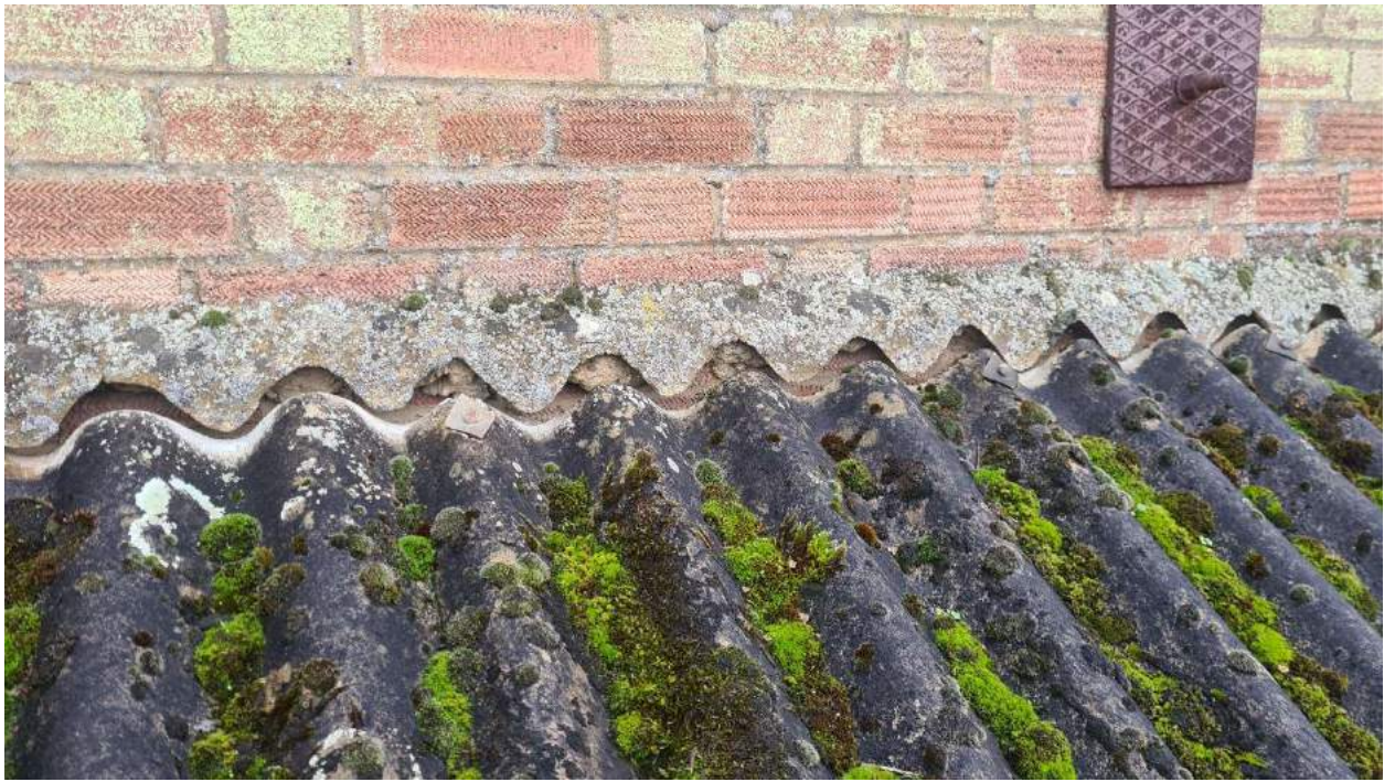
Photograph 5 – Failed lean to roof
