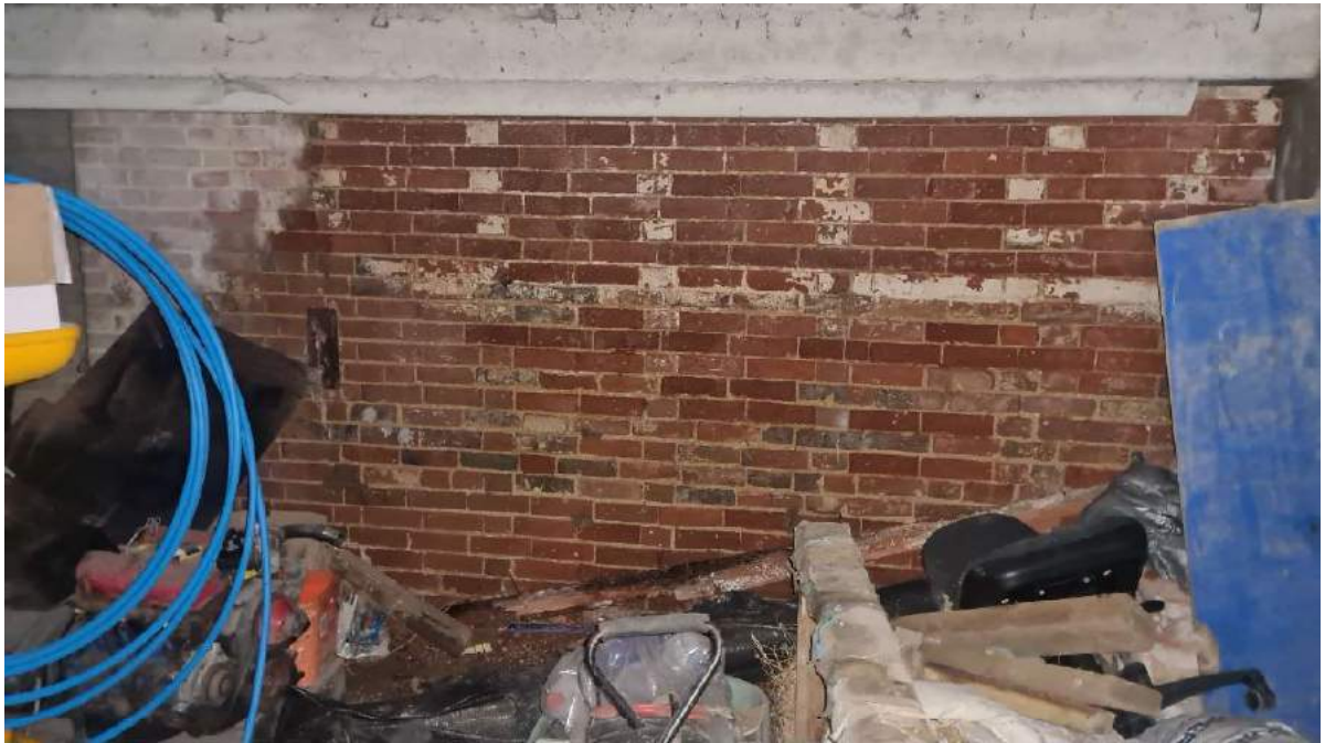
Photograph 11 – Area of water ingress under gutter between Barn A and portal frame shed
