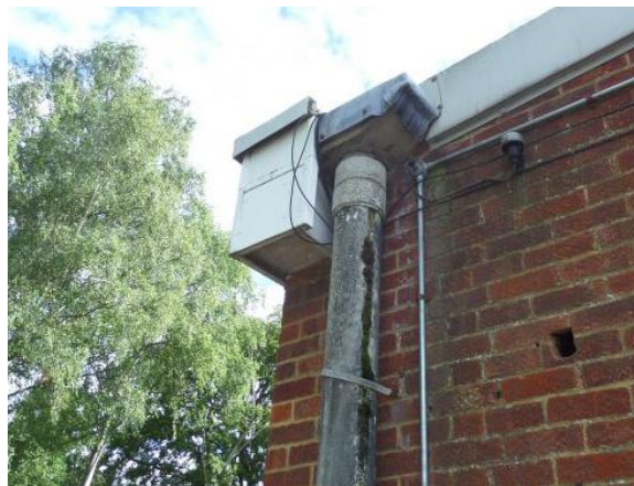
Photograph Two - Possible asbestos down pipe
