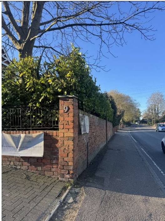
Photo 3: Front Boundary structure exceeding 1.0m in height adjacent to the footpath,
