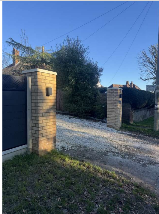
Photo 8: Front boundary structure with brick piers exceeding 1.0m in height
