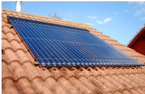
Figure 6: Typical solar thermal panel
