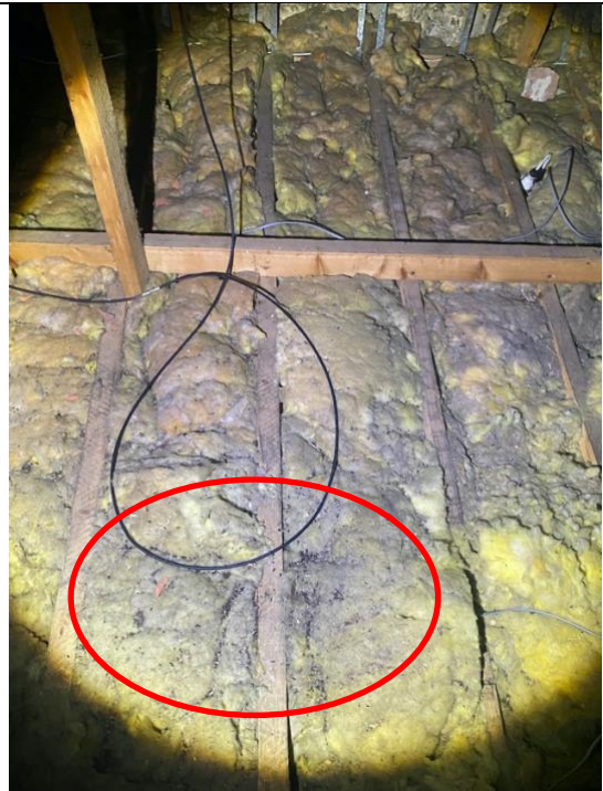
Brown long-eared droppings on floor below the ridge of the roof
