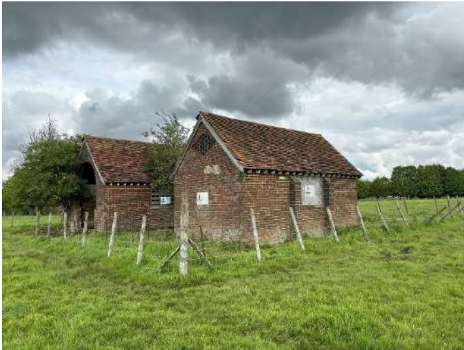
Figure 1: View of the southern corner of the site and dilapidated buildings facing north.
