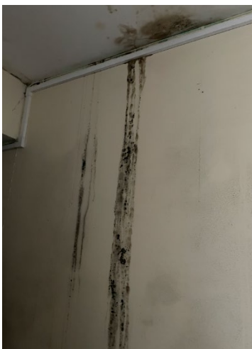
Damp and mould
