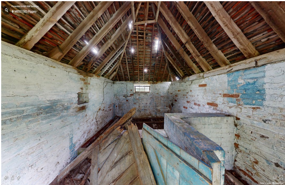
Interior showing the debris including the original boarded door and the poor condition of the brickwork. The enclosure and door on the right is later C20.
