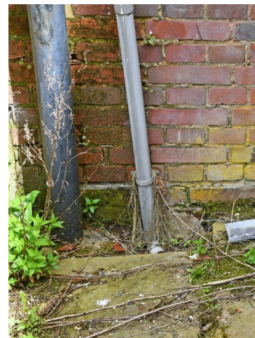
Poor quality and damaged
