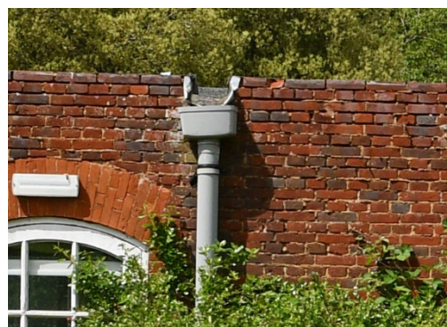
Poor quality details and materials
