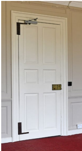
Door and ironmongery
