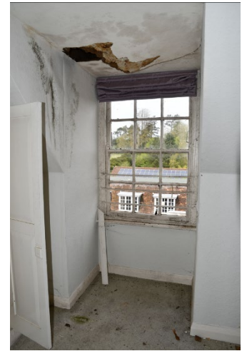
Failure of dormer
