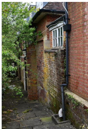
Rear Elevation with damp
