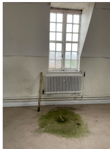
Leaks, damp and mould
