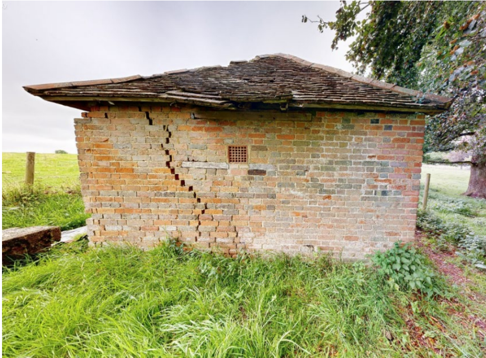
Side elevation showing typical structural movement and poor condition of the roof and eaves. The central section of the roof has deformed and dropped.
