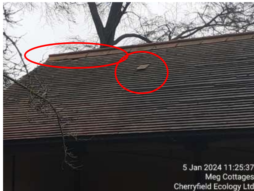
Figure 9: Further examples of gaps within the roof
