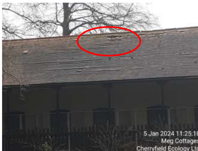
Figure 6: Example of gaps within the roof
