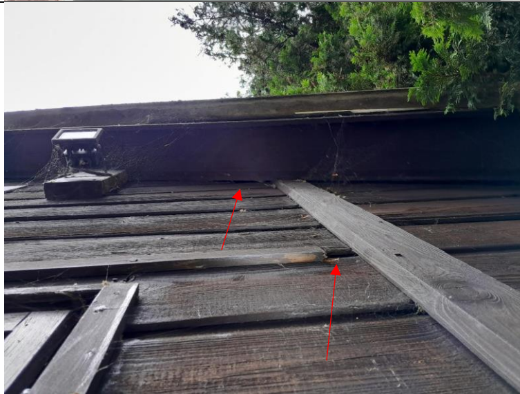
Figure 7 – gaps under cladding and bargeboard on eastern end of B1
