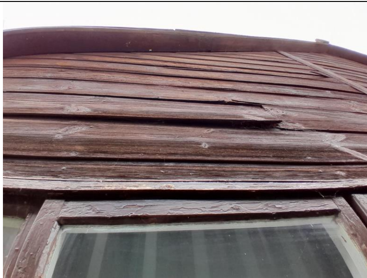
Figure 5 – damaged cladding on western end of B1
