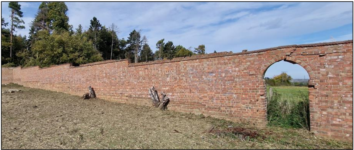
Plate 8: the northeastern boundary wall from the interior of the garden, note the arched doorway leading out to the open field beyond and its structural damage
