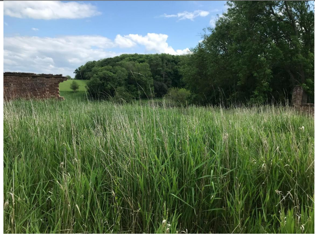
Plate 12: The southeastern wall of the former walled garden has large gaps.
