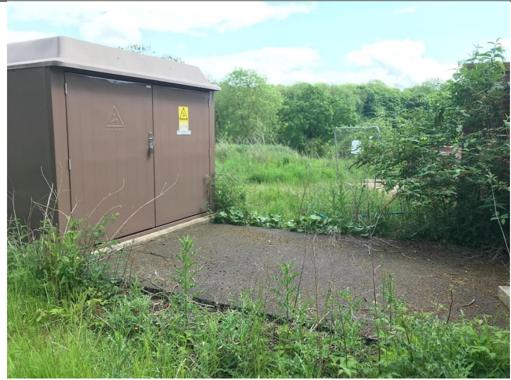
Plate 8: Substation located in northwest part of site.
