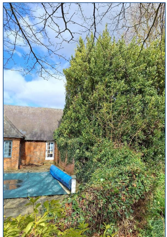
Figure 14: T9 , Bay encroaching on wall
