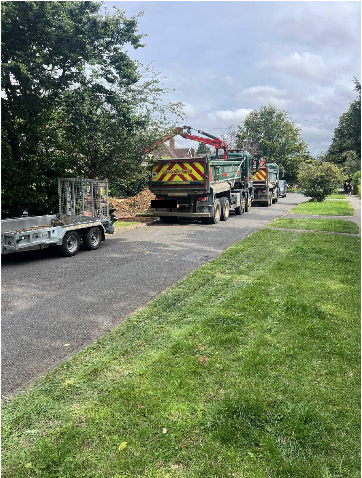
Photograph 3: Highway maintenance convoy — multiple HGVs with crane lorry queued on Cashio Lane during utility works. Demonstrates routine use of the lane by heavy vehicles and the impossibility of safely reversing onto it.
