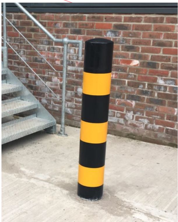
Example: Protective Bollard
