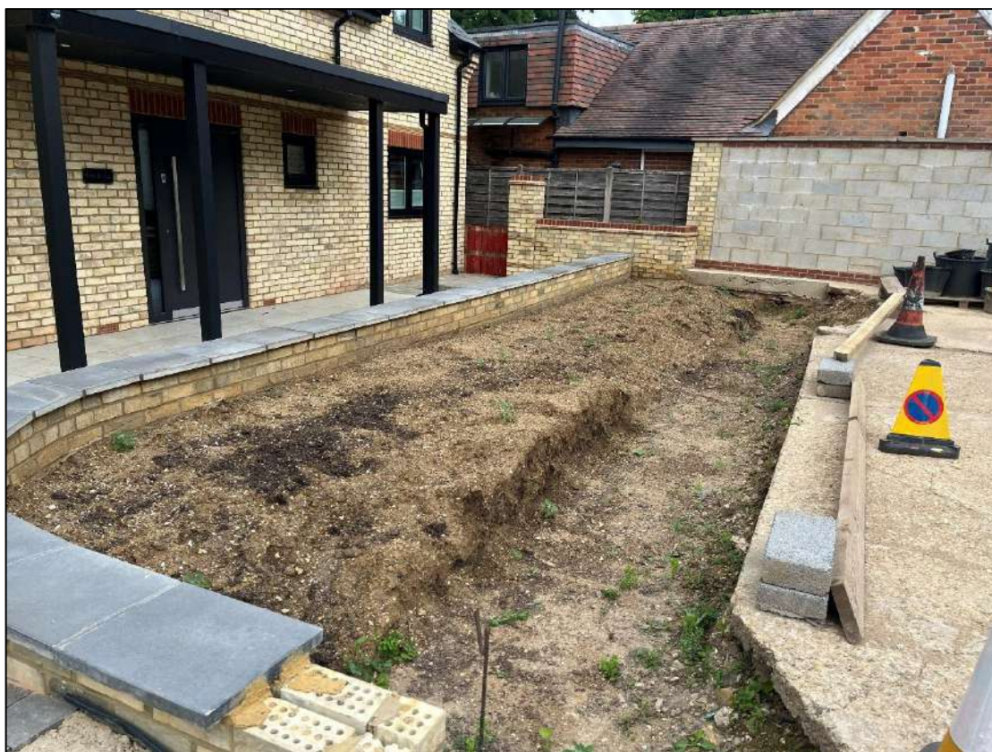
Figure 4: View of bare ground along the northern boundary.
