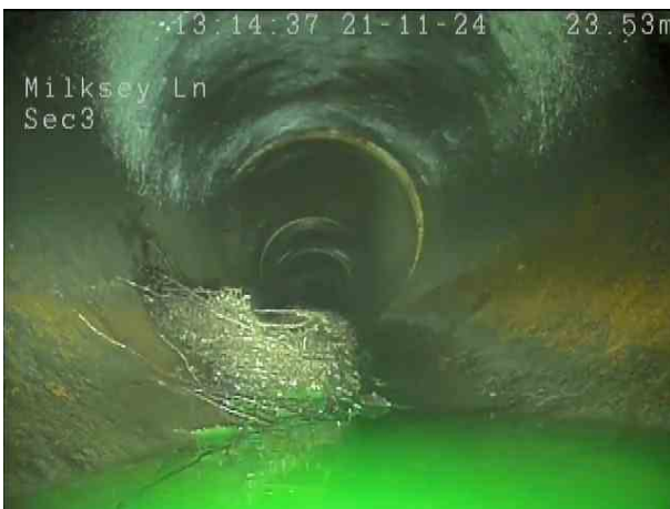
f4683594-3657-44ac-96e9-ee69abbc467a.png, 00:02:37, 23.80 m Roots, mass, 10% cross-sectional area loss, start
