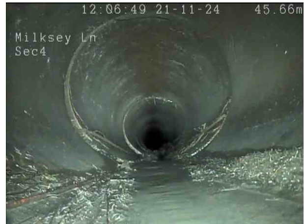
79ca1f7a-4d21-486e-864e-0eff7670a4b5.png, 00:04:17, 45.70 m Roots, mass at joint, 5% cross-sectional area loss, change
