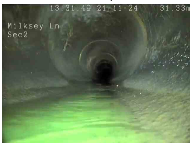
6587682b-d075-46d0-bbc0-423006ded360.jpg, 00:02:45, 31.30 m Finish node, other special chamber, reference: SW2, Cross
