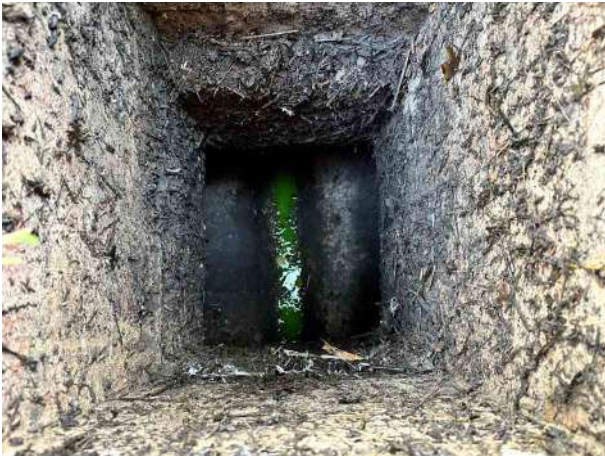
SW3.JPG, 00:00:01, 0.00 m Start node, inspection chamber, reference: SW3
