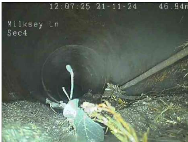
5aaf0228-9991-490b-b1c3-98dcc6b319a3.png, 00:04:52, 46.90 m Roots, mass at joint, 20% cross-sectional area loss, change
