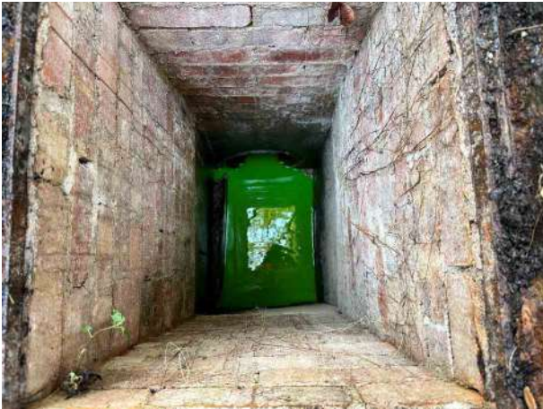
SW4.JPG, 00:00:01, 0.00 m Start node, inspection chamber, reference: SW4
