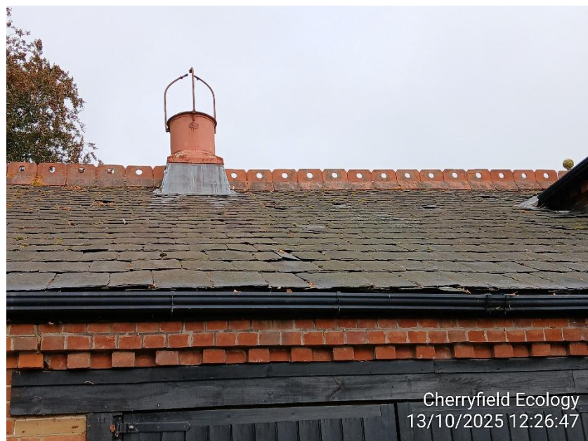
Figure 36: Example of gaps around tiles.
