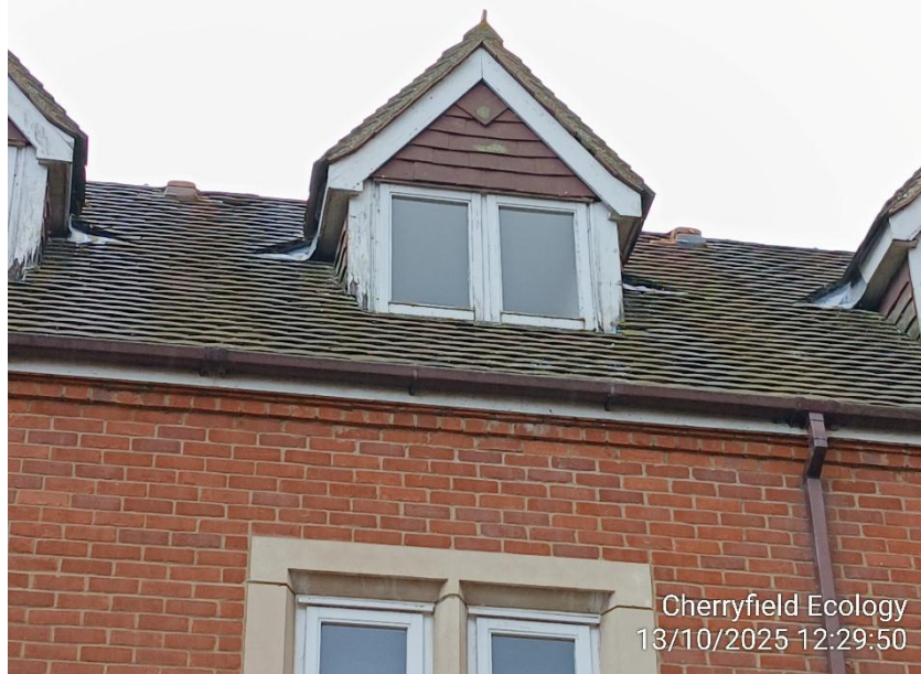
Figure 33: Example of gaps around tiles.
