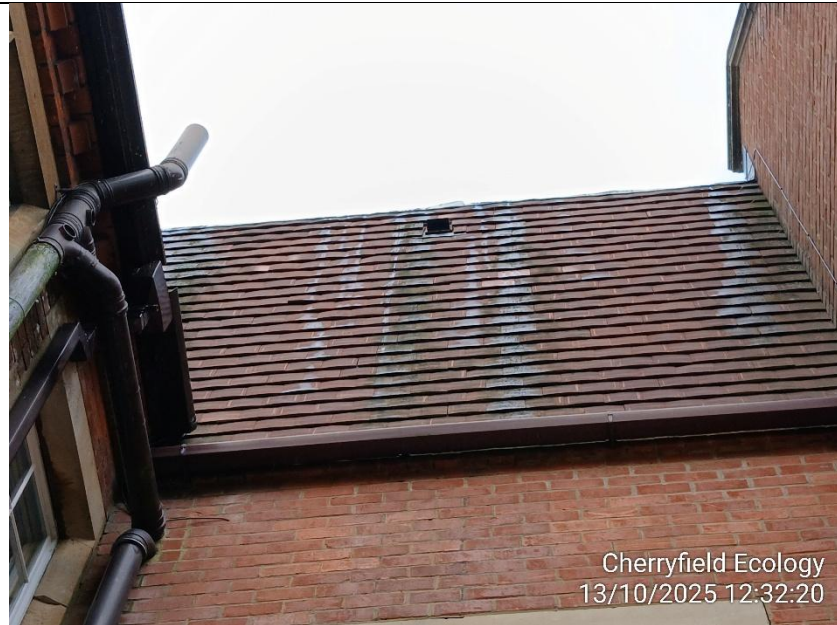
Figure 35: Example of gaps around tiles.
