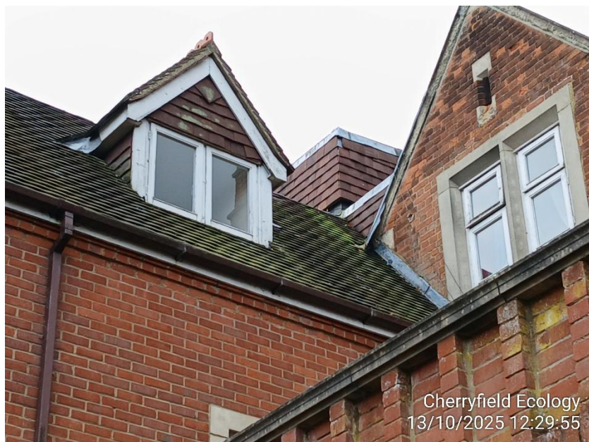
Figure 34: Example of gaps around tiles.
