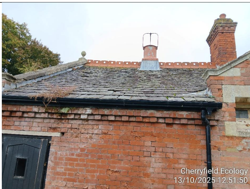
Figure 37: Example of gaps around tiles.
