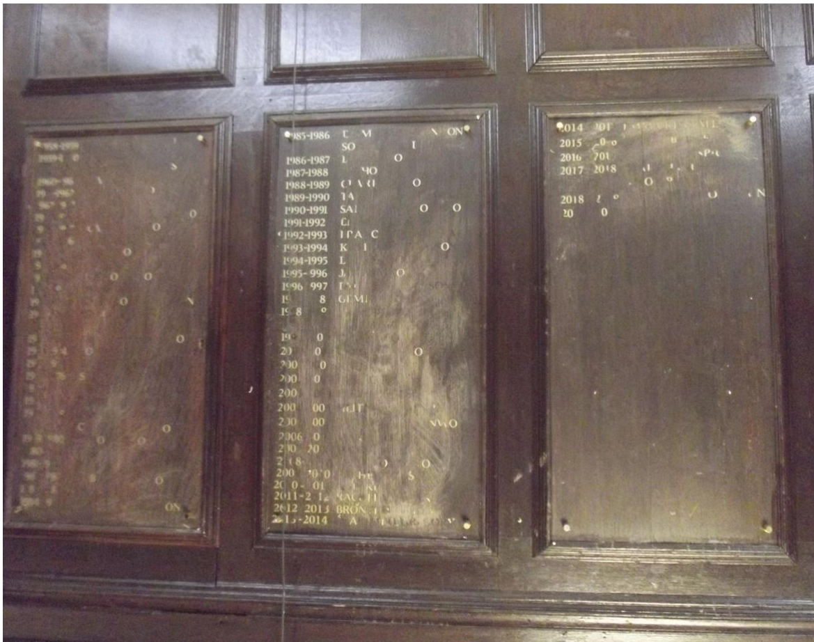
77. School Hall honours boards with damaged lettering
