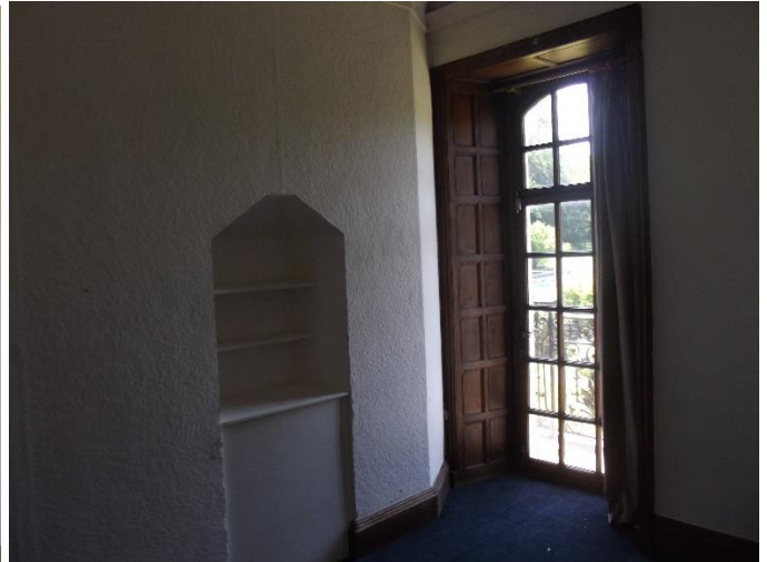
59. Wall cutting through former bedroom
