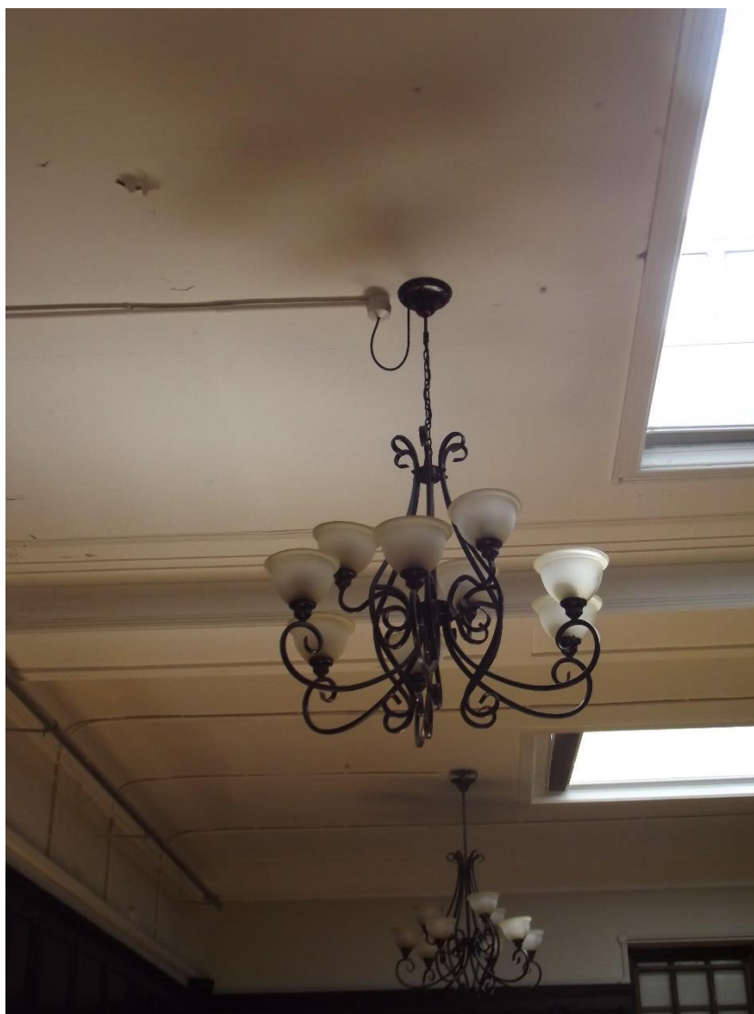
79. Hall light fittings
