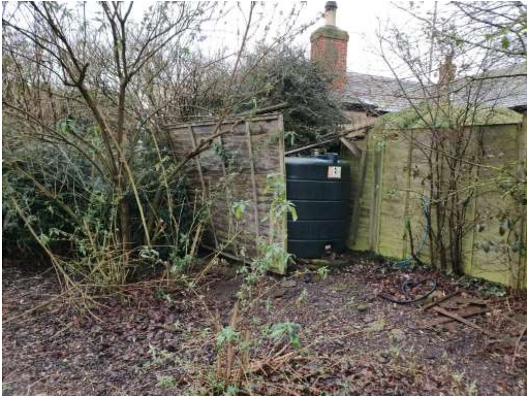
Photo 9: Heating oil tank adjacent to residential building facing south-west.
