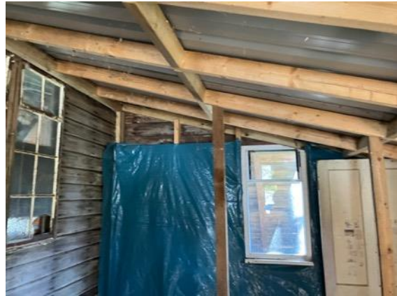
Photograph 2: Building B1b - timber workshop extension against timber wall of building B1a with broken window, metal roof and some insulation
