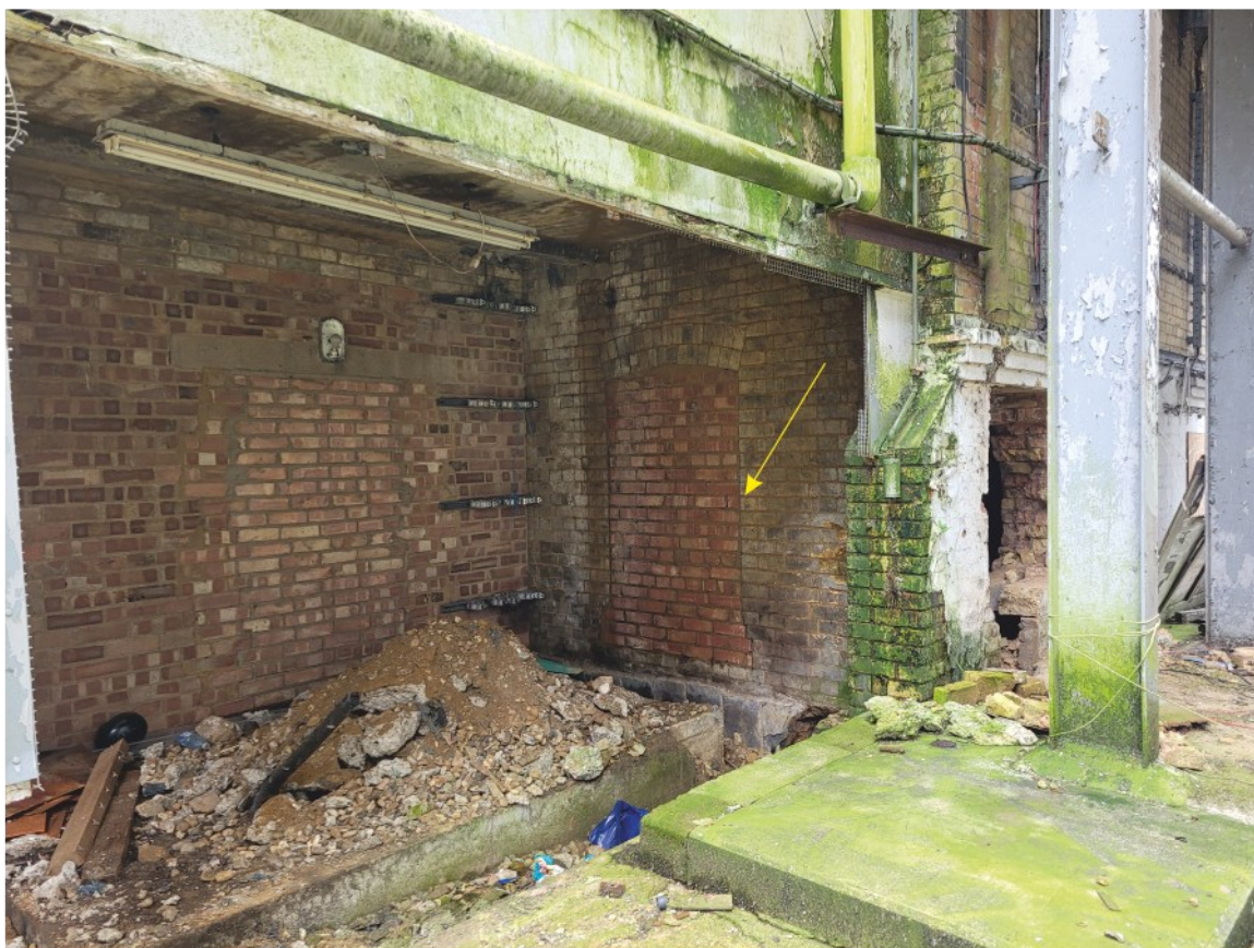
Pl. 22 Blocked door at north end of north elevation of roller mill
