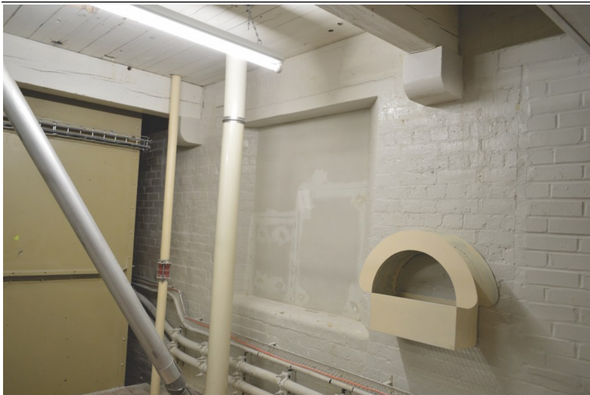
Pl. 39 Second floor blocked window and corbel supporting ceiling joist on north wall. 2017 (N. Field)
