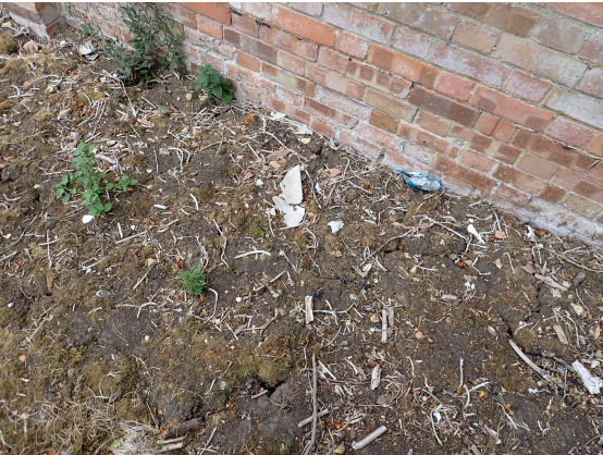
CEMENT SHEET FRAGMENTS INSIDE EASTERN CURTILAGE
