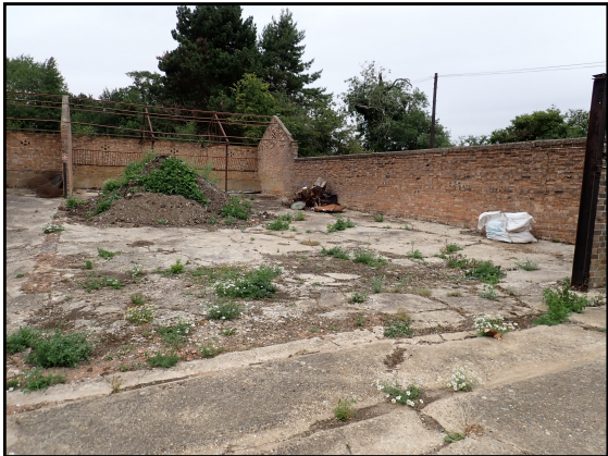
SPOIL HEAP ON CATTLE SHED FLOOR SLAB
