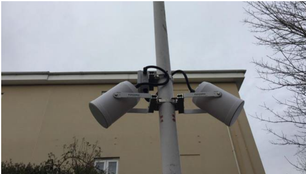
Figure 3 - Installed speaker system (GTR, December 2024)
