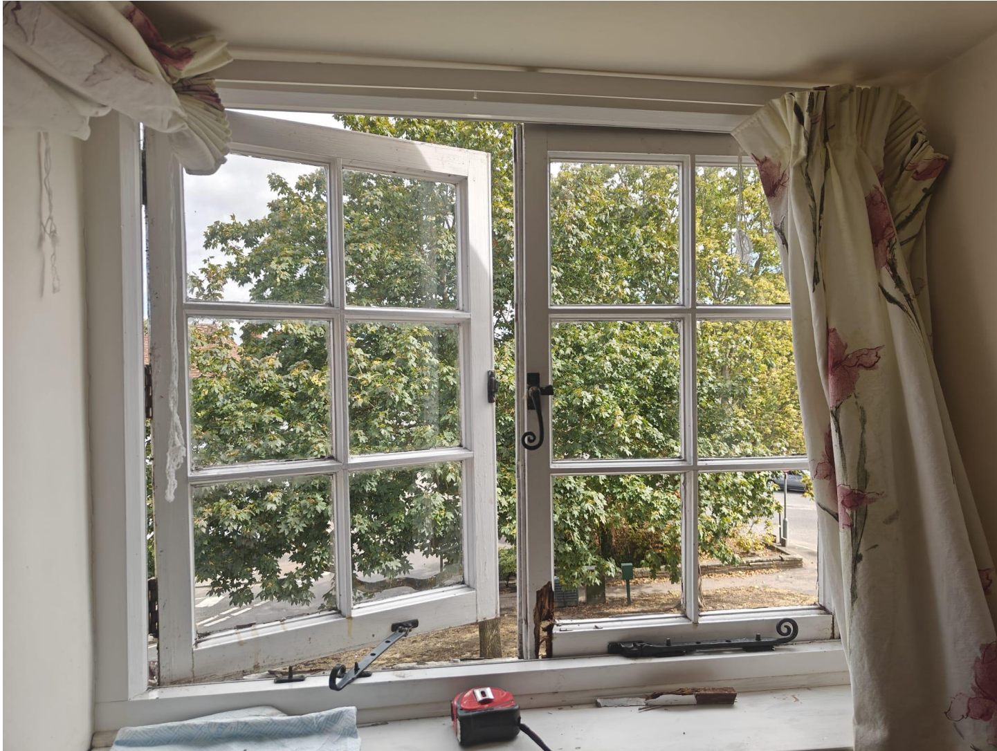
Rotten and broken window in Child bedroom
