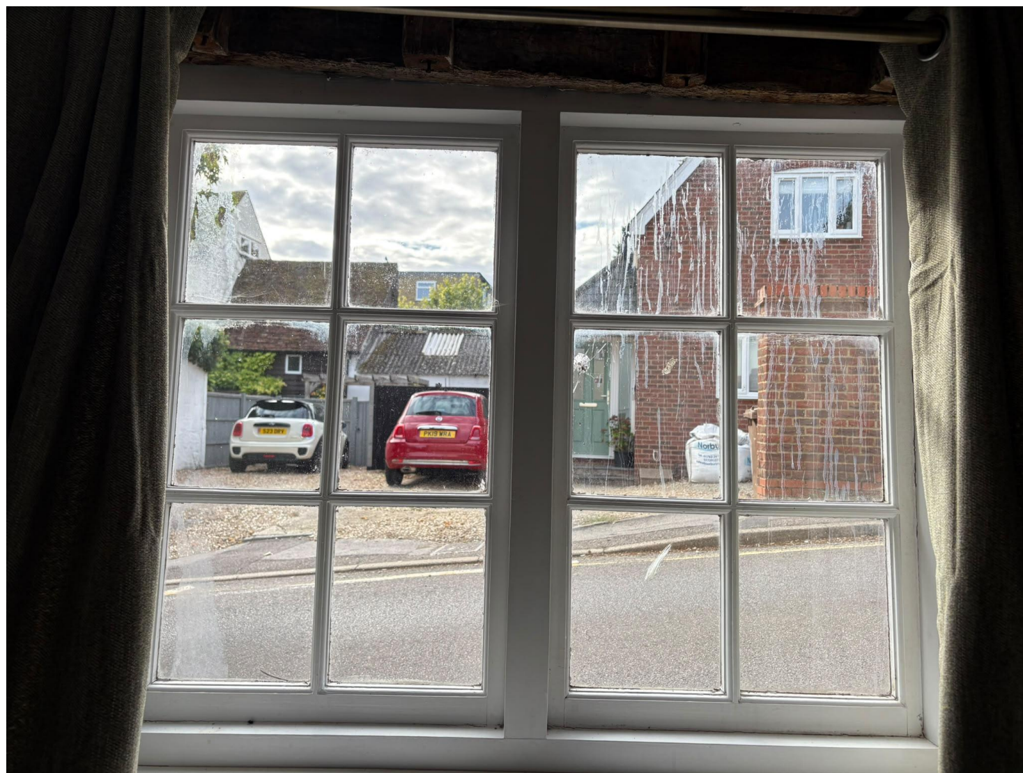
Window 6 showing damage.
