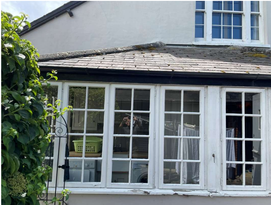
Existing casements sitting proud of the surrounding frames
