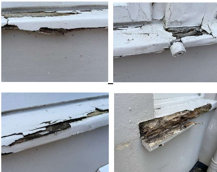
Existing windows with rot setting in
