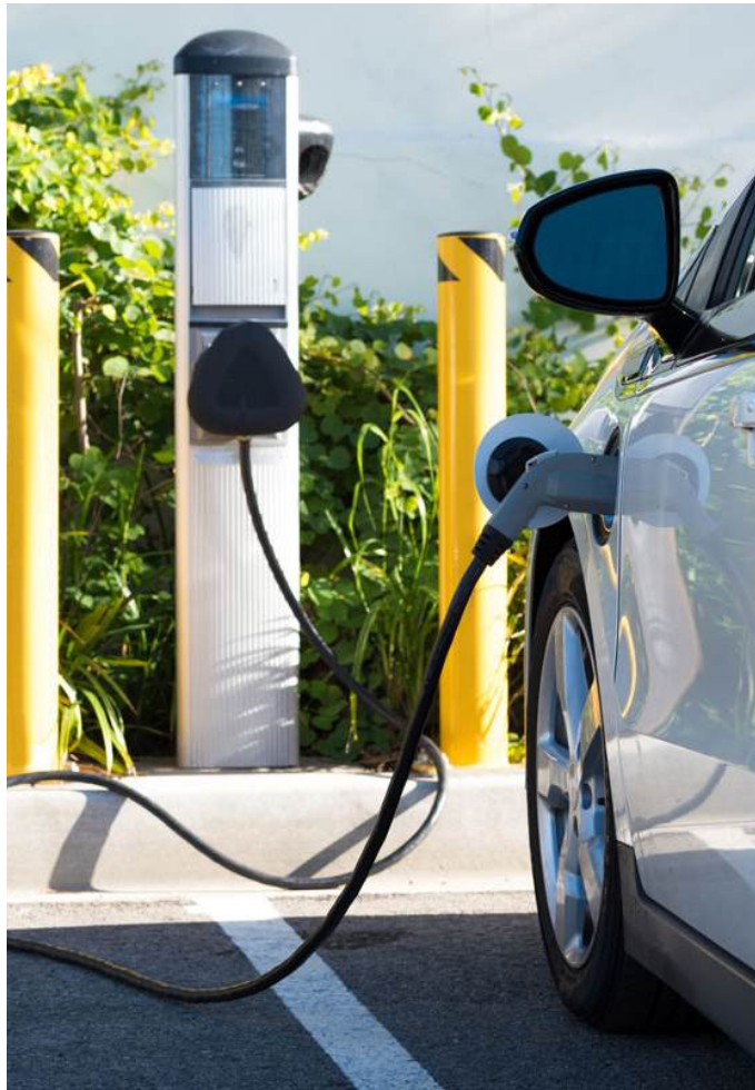
Typical image of electric car charging points to all units.
