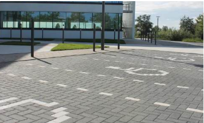
Permeable Block paving to car parking bays with contrasting demarcating blocks
