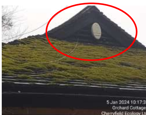
Figure 7: gaps within the louver
