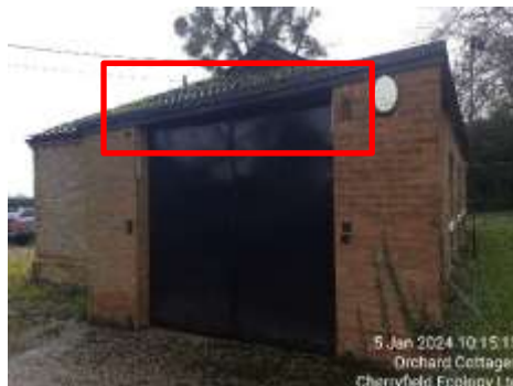
Figure 6: gap under the doorframe
