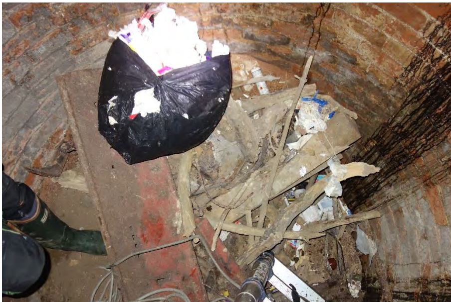
Photograph 13: Ice House No. 2 – waste at the base of the chamber
