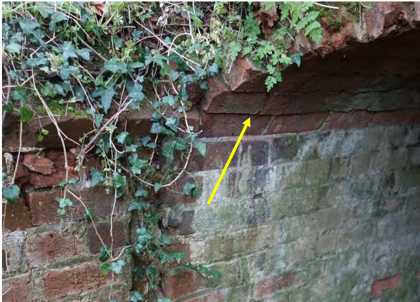
Photograph 5: Slight displacement of brickwork at the arch springing point (arrowed)
