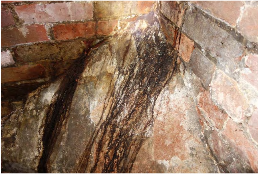
Photograph 12: Staining due to water ingress (typical example).
