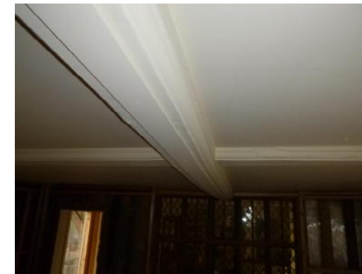
Beam at living room ceiling sags in line with sloping and sagging floor above (5)
