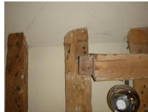
Detached tenon at end of purlin - historic damage (16)
