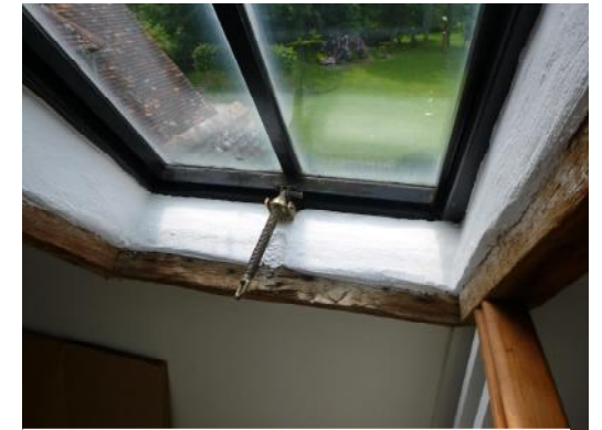
Roof window, with some signs of condensation
