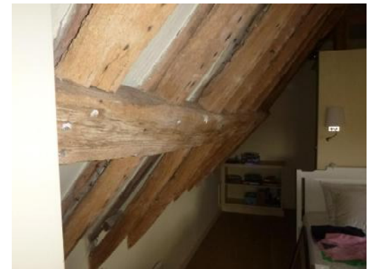
Rear (north) purlin sags due to removal of collars and relocation above head height (13)
