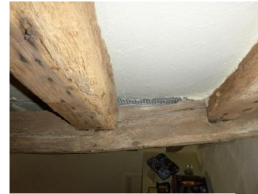
Gap between purlin and ceiling, judged historic with no sign of recent movement (13)
