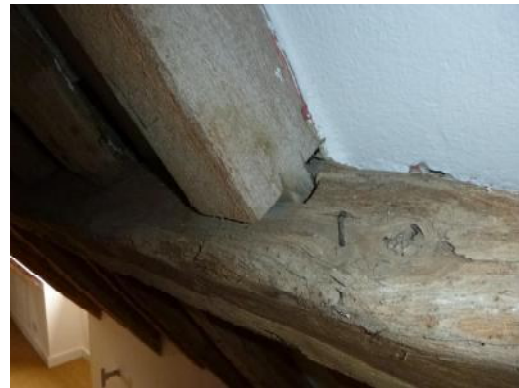
Rafters tenoned into purlin, with wrought iron repair strap below - historic (5)
