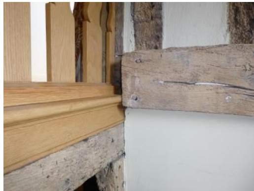
Side rail of stairwell tower meets landing at slightly higher level
