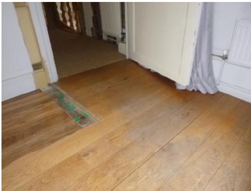
Entrance to bedroom - floor slopes away from here (2)
