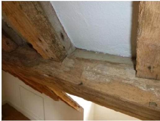
50mm gap between purlin and ceiling - no sign of recent movement (7)
