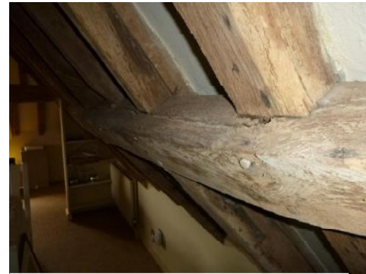
Historic sag to purlin (13)
