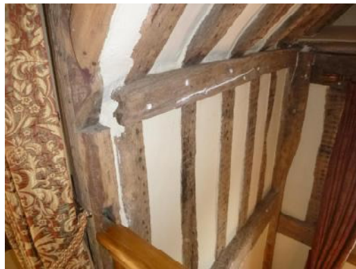
Eaves rail detached from post due to historic rot damage (5)
