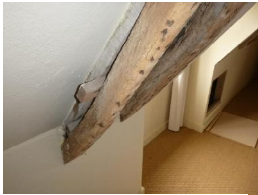
Sagging rafters packed out (13)
