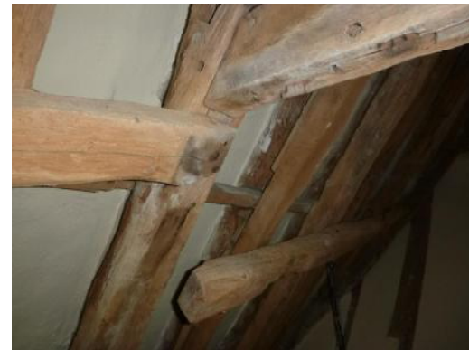
Detached purlin and sagging rafters, packed out roof profile - judged historic (22)
