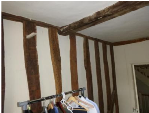
Spine beam over bedroom, meets wall not in line with studs. Considered OK, relying on tenon joint to head rail.
