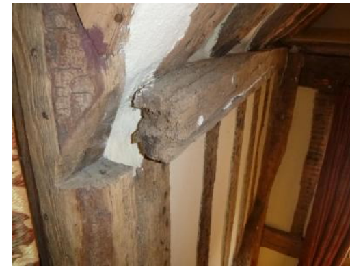
Detail of eaves rail - no sign of recent movement (5)
