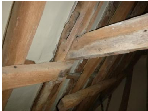
Gable frame with empty mortise and detached purlin (22)
