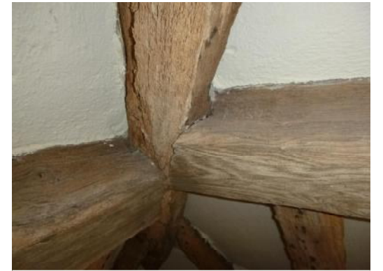
Purlins meet at hip - historic damage (17)
