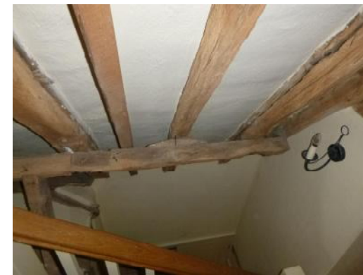
Unsupported end of east purlin, which cantilevers towards wall of SE wing. Supported by strut from house wall (19)
