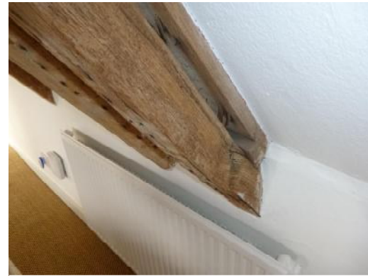
Gap between rafters and ceiling, with packing (7)
