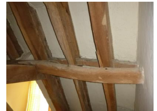
Historic distortion of purlin adjacent to collar and dormer
