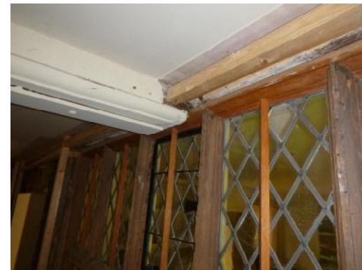
Spine beam bearing on window head is structurally illogical, but not unique
