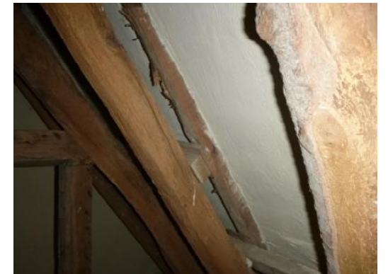
Sagging rafters packed out to restore roof profile - judged historic
