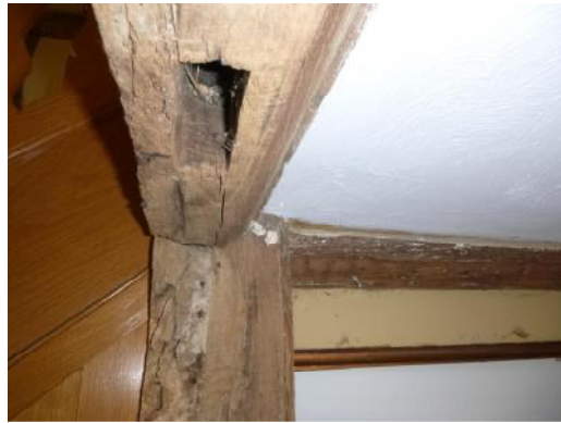
Empty mortise in headrail (4)
