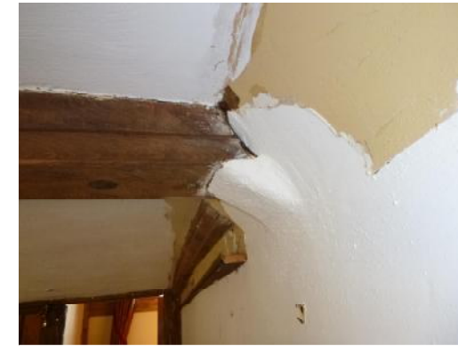
Repair at bearing in chimney - appears to be holding but potentially suspect. Investigation recommended
