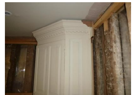
Cupboard in corner has been relocated and is mounted on an OSB backing
