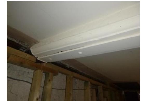
Steel strap beneath beam is ineffective as many more screws would be needed to transmit shear forces effectively
