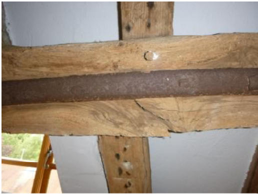
Fracture in front purlin, repaired with strap - judged historic (5)
