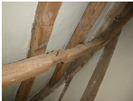
Inward sag of purlin (22)
