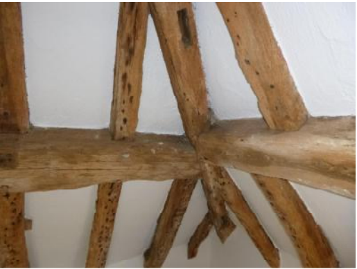
Empty mortises in hip beam suggest previous alterations (1)
