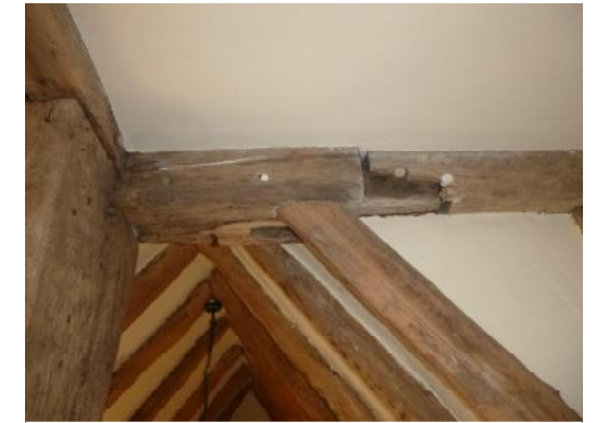
Historic damage to scarf joint in head plate, plus empty mortise (4)
