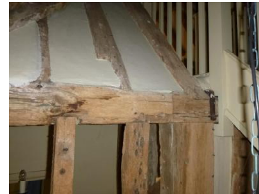
Head rail of house wall, showing witness of water damage - judged historic
