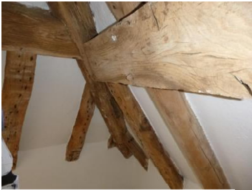
Empty mortises suggest previous alterations to roof (1)
