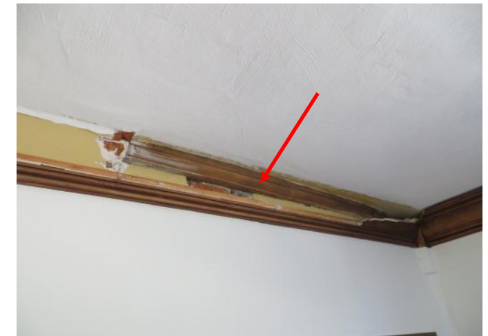
Figure 4.196: Showing an original 17th century cornice (marked in red) revealed.
