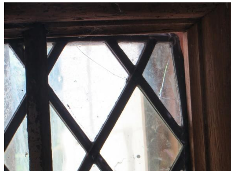
Figure 6.1: Showing an example of the broken glass panes in the historic leaded light casement in the existing dining room.
