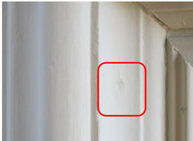
Figure 4.202: Showing a screw hole infilled with filler.
