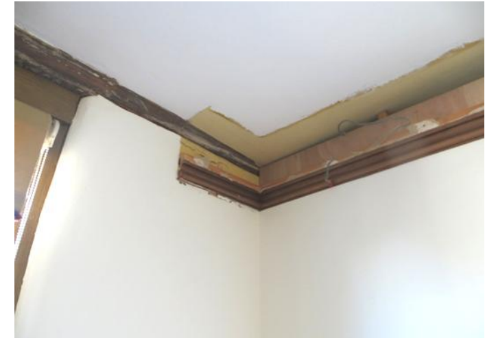
Figure 4.194: Showing the part of the historic cornice above and the modern cornice below (latter prior to removal).
