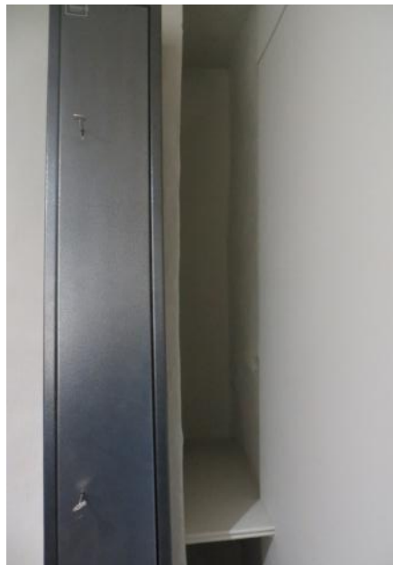
Figure 4.141: Showing the void between the chimneystack and the western wall of the dressing room.
