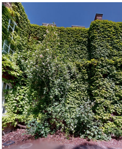
Stable Block South Elevation – vegetation shall need to be removed and extensive repointing carried out.
