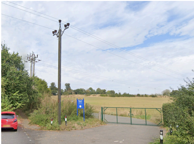
Overhead cables on site
